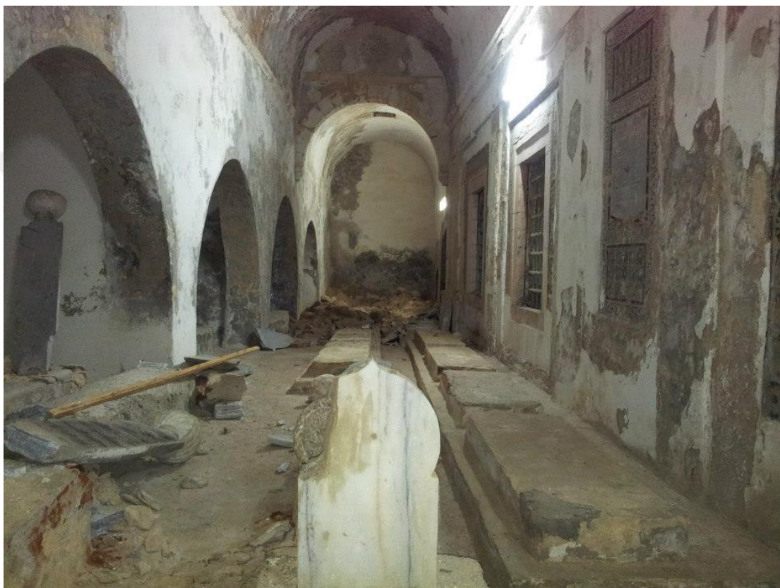
Figure 3. 60: The Vandalism and Destruction of the Cemetery in Ahmed Pasha Mosque
