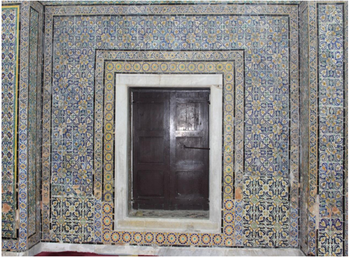
Figure 3. 49: General Picture of the Decoration the Ceramic Also Shows a Detail of the Windows and the Northern Entrance to the Mosque
