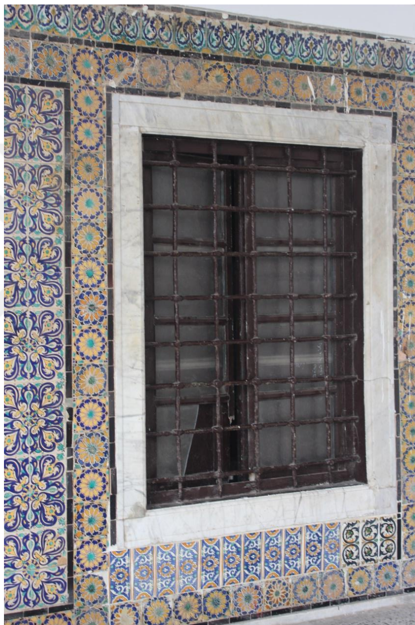
Figure 3. 48: The Front Faced of the Window With the Coating of Ceramic Pieces (Source: by the researcher)
