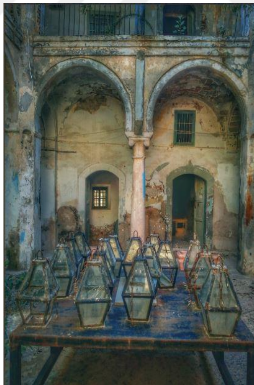
Figure (B) A photo collection showing the bad Ahmad Basha Garramanli School situation
