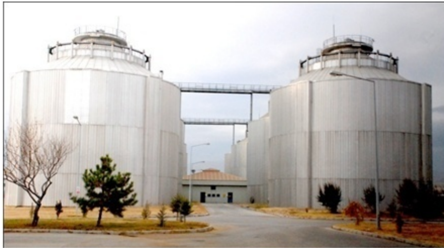
Figure 3. 7: Photograph of anaerobic digesters.
