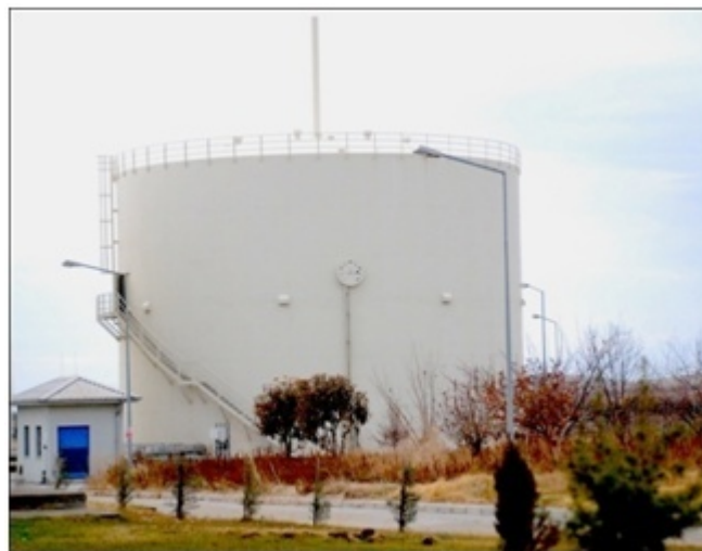
Figure 3. 8: Photograph of biogas storage tanks.
