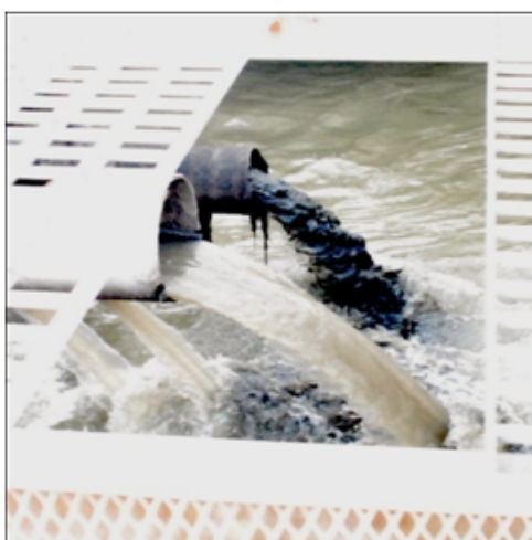
Figure 3. 9: Mixing point of recycle stream influent at ACWTP.
