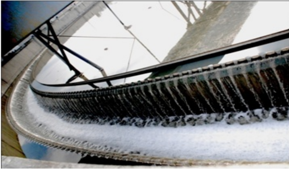
Figure 3. 4: Photograph of primary clarifier.
