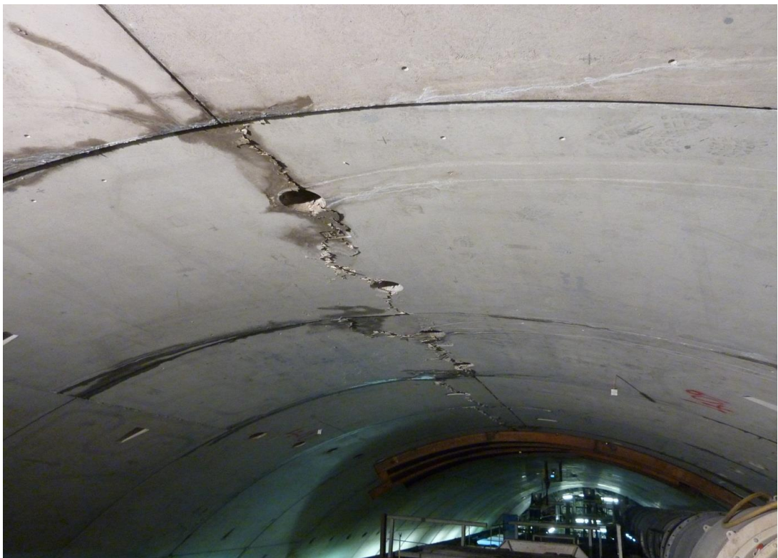
Figure 6.8 : Cracks on the segments.
