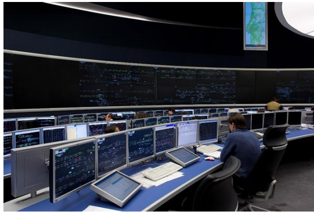
Figure 2.1: A Train control center (TCC) and Dispatcher [9]
