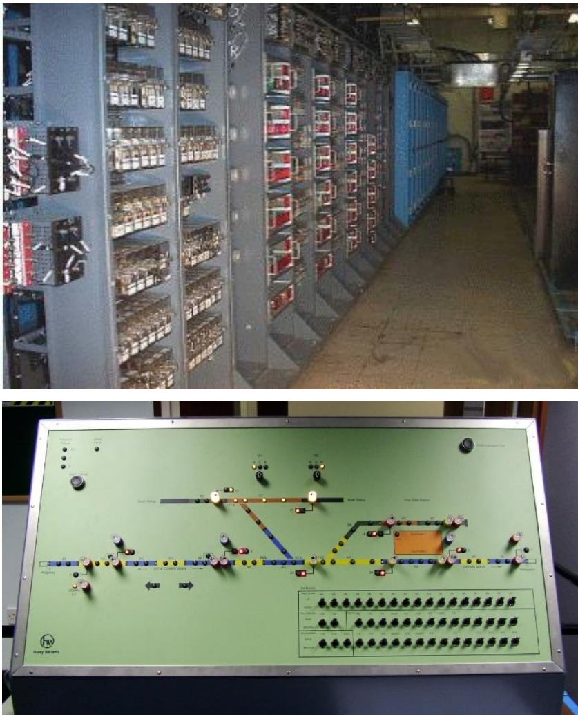
Figure 3.2 : A relay interlocking system and a control panel [24].
