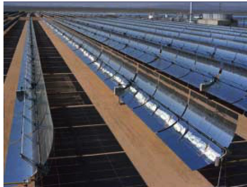
Figure 1.1. Trough Collector Field in Kramer Junction, California.
