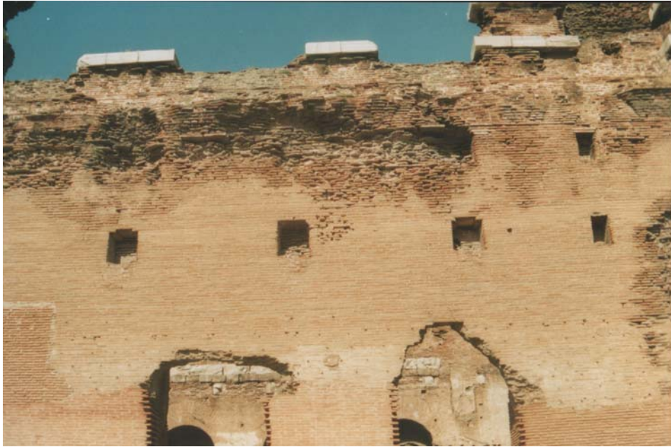
Figure 4. 97. Loss of material in the south-west elevation (2004)
