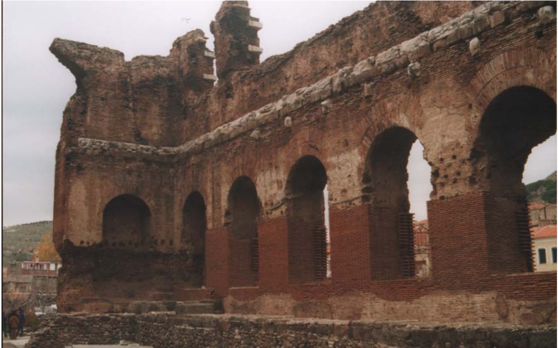
Figure 2. 14. An interior view of the restoration sections of the structure carried out in 1940s in the Serapis Temple (2004).
