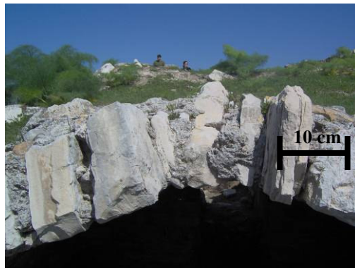
Figure 3.13. Break out due to constructional cause
