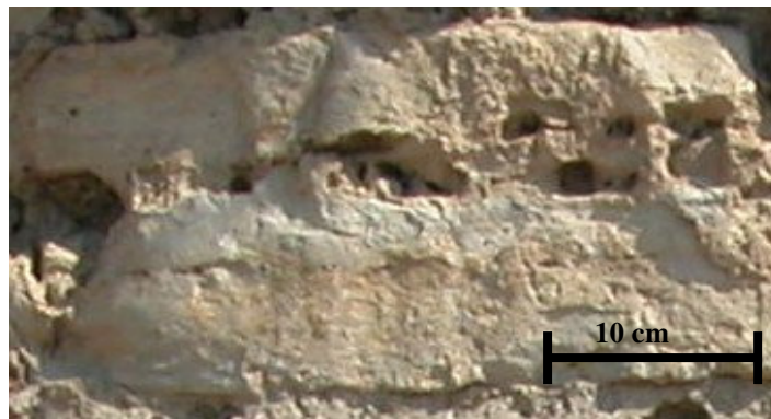
Figure 3.9. Weathering out of stone components
