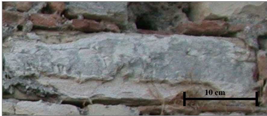
Figure 3.3. Back weathering due to loss of crumbs/splinters
