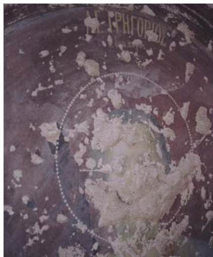
Figure 5.38. Loss of plaster and painting layer due to dampness in the painting no:4 on the main apse of the church
