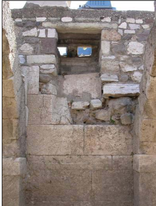
Figure 3.53. The present situation of the east wall and the windows.
