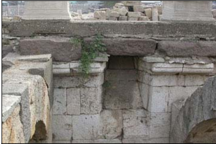
Figure 4.18. Fourth course of the wall with cyma reversa moulding is displayed in a restricted area.
