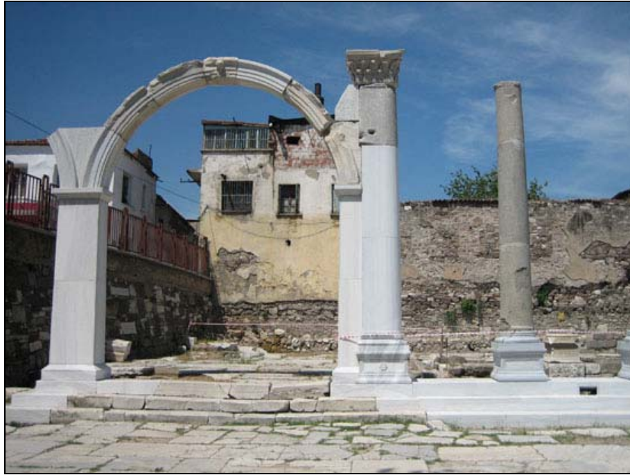
Figure 4.46. Reconstruction implementation of the West Gate and the 30 th column of the West Soa.
