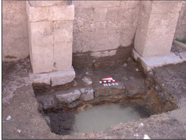
Figure 4.20. The sounding work between 4 th and 5 th axes reveals the foundation of the wall. (Source: Archives of the Agora excavations, 2004)
