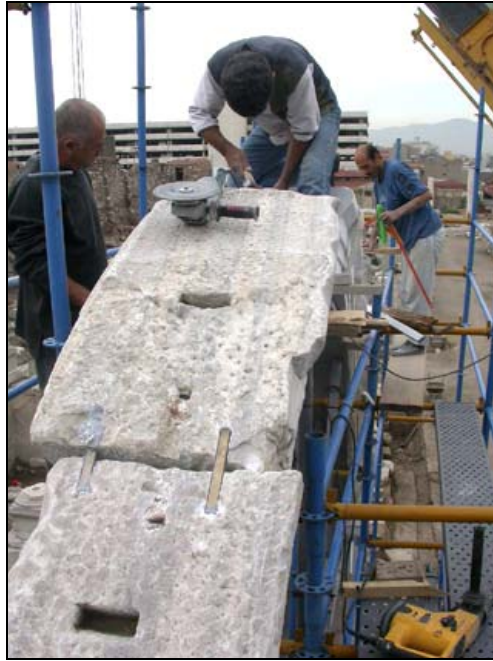
Figure 4.12. Upper face of the voussoirs; dovetail cuts, original clamp place and applied bronze clamps are seen. (Source: Archives of the Agora excavations, 2004)
