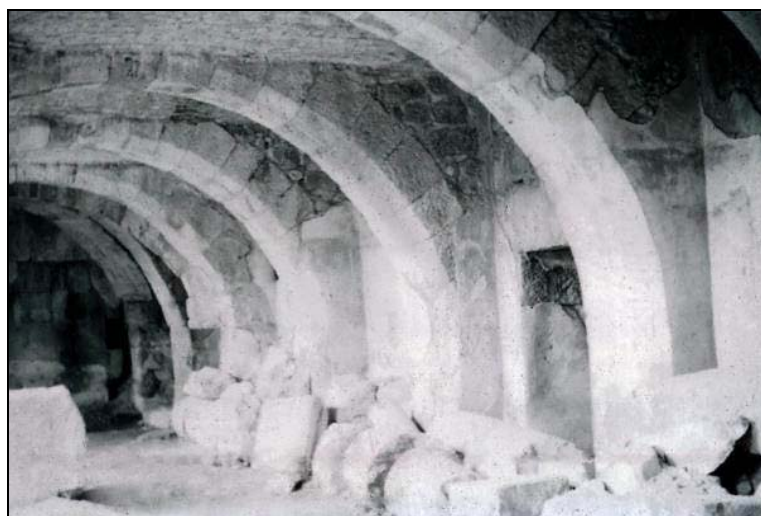
Figure 3.50. The plasters seen on the walls in December 1961 do not exist today. (Source: WEB_24 2006)
