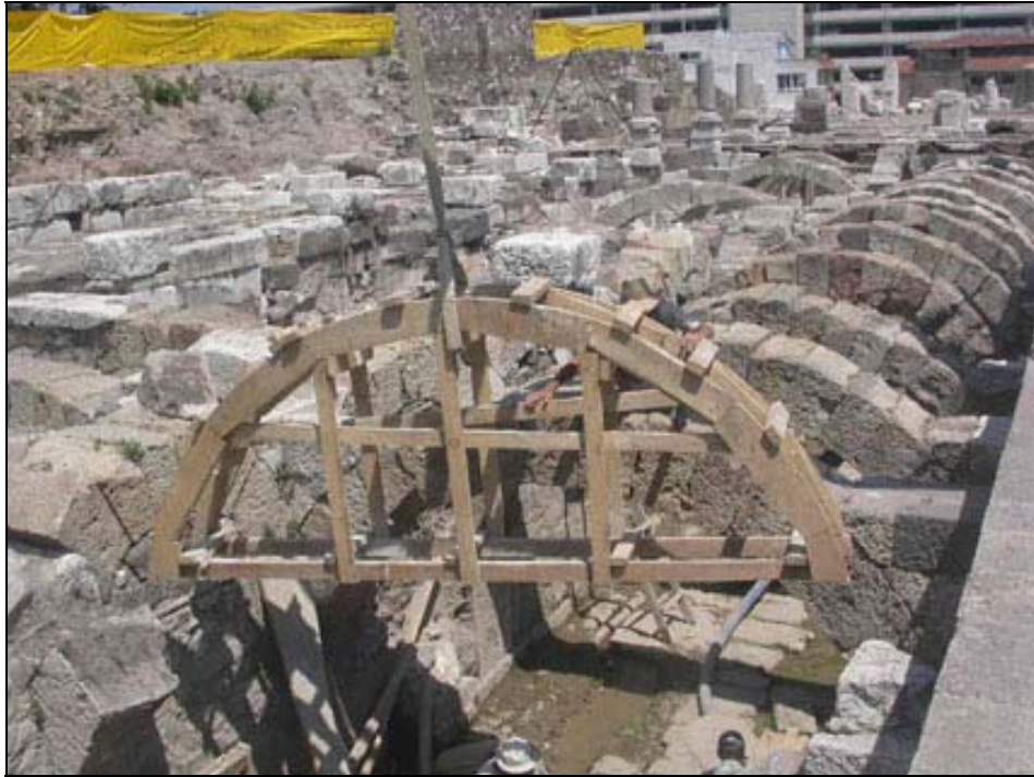
Figure 4.41. The timber staging is placed initially. (Source: Archives of the Agora excavations, 2005)
