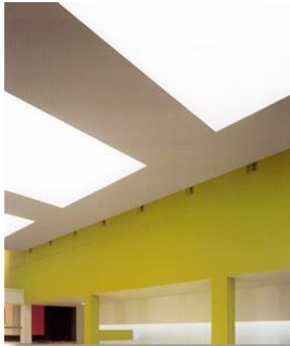
Figure 3.6. The use of transparent PVC sheeting in the ceiling.
