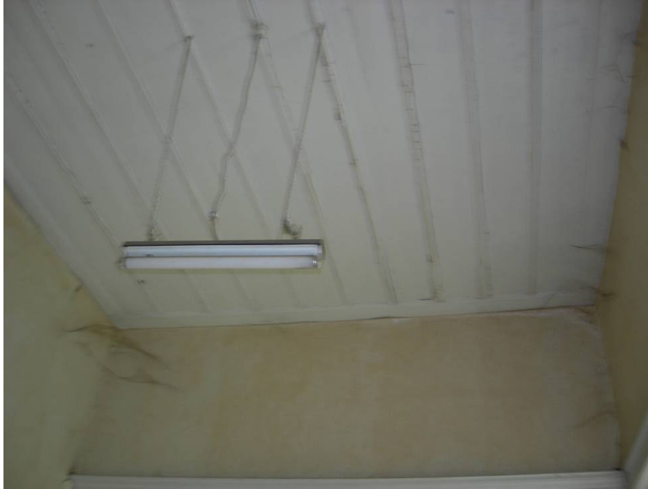
Figure 2.46. The ceiling covering of room 3.
