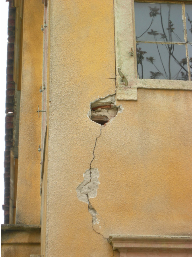
Figure 2.118. The major crack at the bottom level of the window at the northern corner of the western facade.
