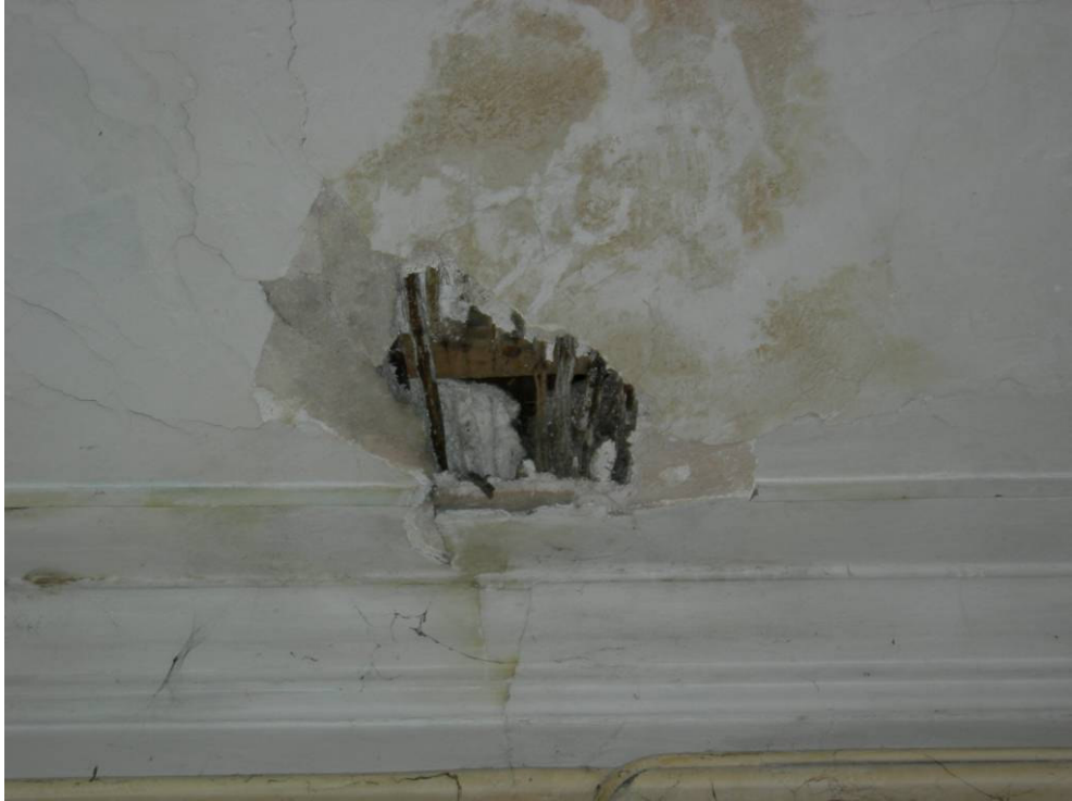
Figure 2.136. The deteriorated plaster and wood laths of the ceiling of the hall at the first floor.
