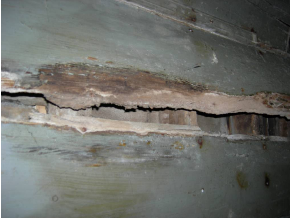
Figure 5.6. The deteriorated ceiling coverings that are suggested to be removed.
