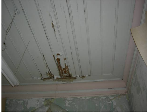
Figure 5.8. The deteriorated wood laths that are suggested to be removed.
