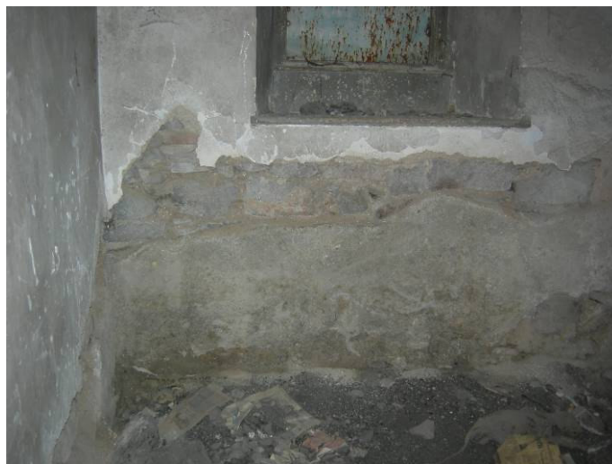
Figure 2.16. The loss of plaster observed on the bottom parts of the walls at the basement.
