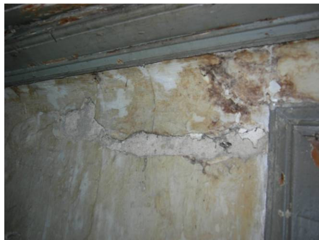
Figure 5.5. The deteriorated plaster that is suggested to be replaced with plaster in original composition.
