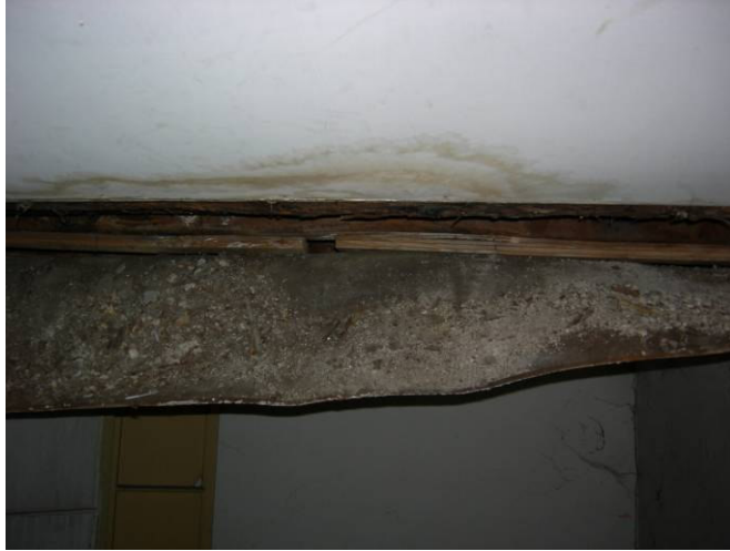
Figure 5.3. The plywood ceiling covering of storage space at the mezzanine floor that is suggested to be removed.
