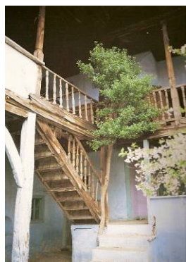
Figure 3.66. The simple stairs with single flight parallel to the open hall. (Source: Kuban 1995)
