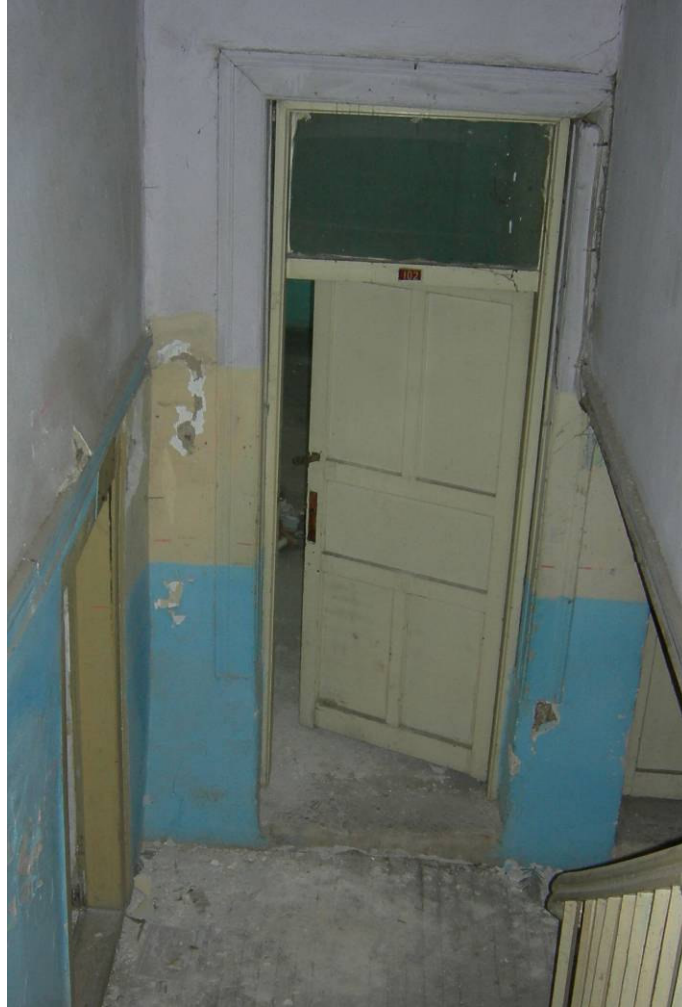
Figure 2.58. The door of the room 2 of the annex at the mezzanine level.
