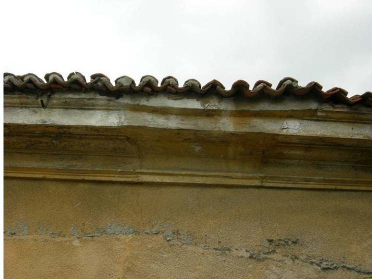
Figure 4.16. The trace of the fireplace at the eastern facade of the house.
