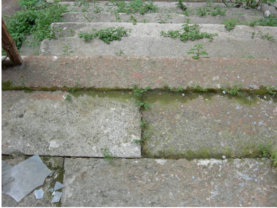
Figure 2.128. Microbiological growth on the stone coverings of the northern terrace.
