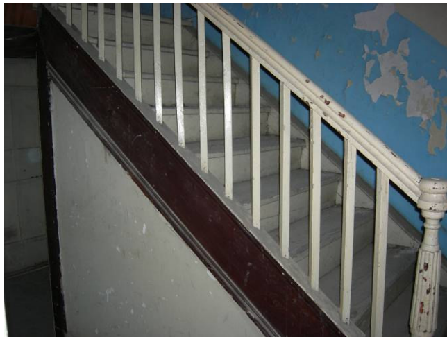
Figure 5.4. The unqualified timber balusters that should be removed.
