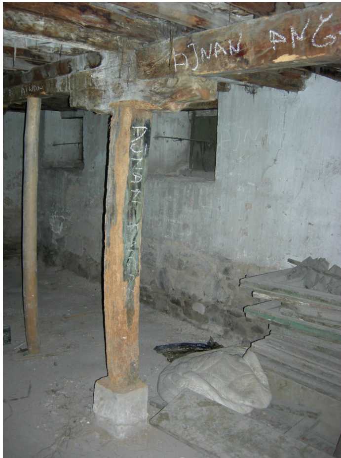
Figure 2.121. The timber beam at the basement which has deflection towards the middle.
