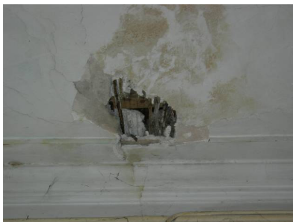
Figure 5.10. The plaster and the deteriorated wood laths that are suggested to be removed.
