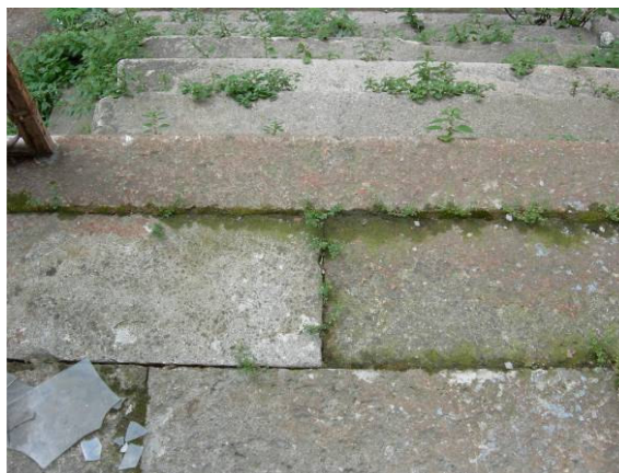
Figure 5.13. The rust stains on the stone that are suggested to be cleaned.
