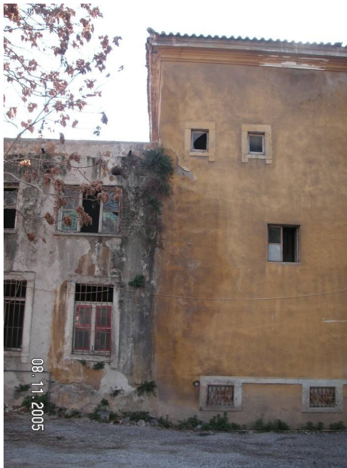
Figure 2.89. The windows of the service spaces at first and mezzanine floor levels.
