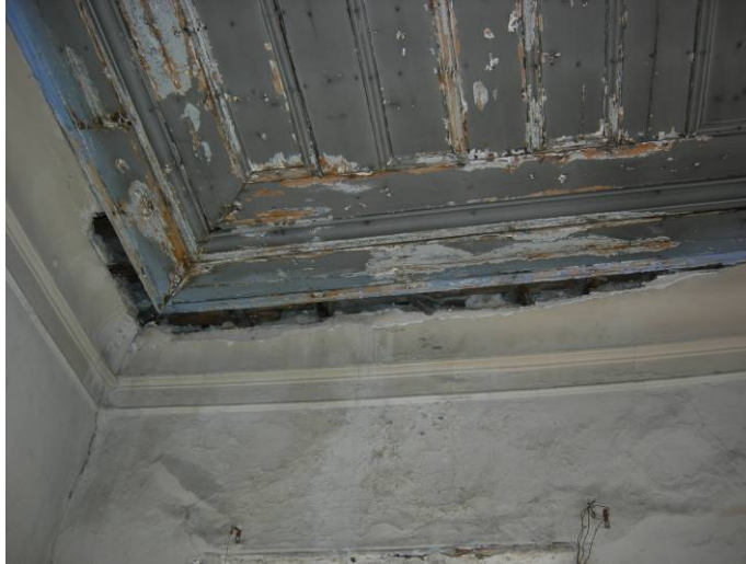
Figure 5.11. The deteriorated timber coverings that are suggested to be replaced.
