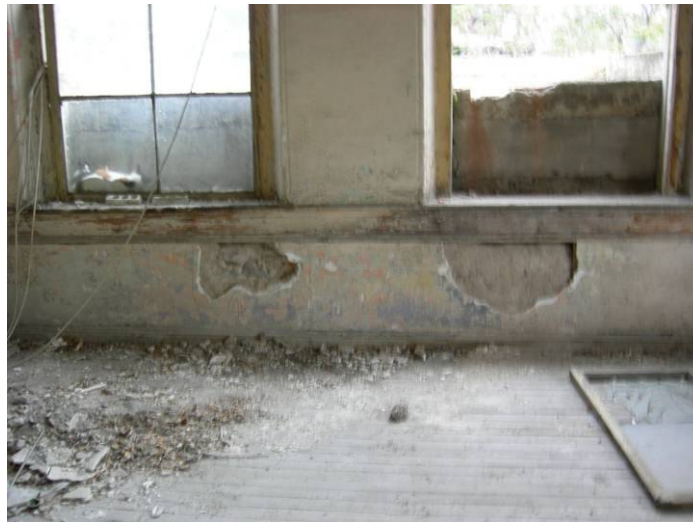
Figure 5.12. The deteriorated plaster on the east wall of room 6 that must be replaced
