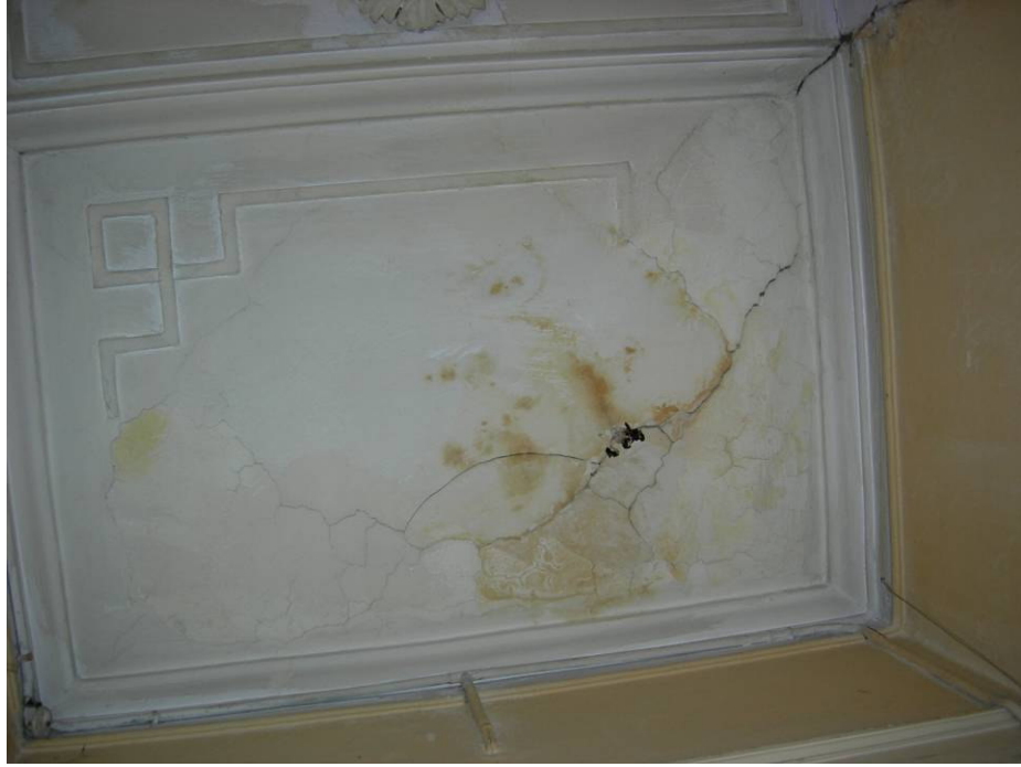
Figure 2.134. Cracks and discoloration in plaster of the ceiling of the stair hall at the first floor level.
