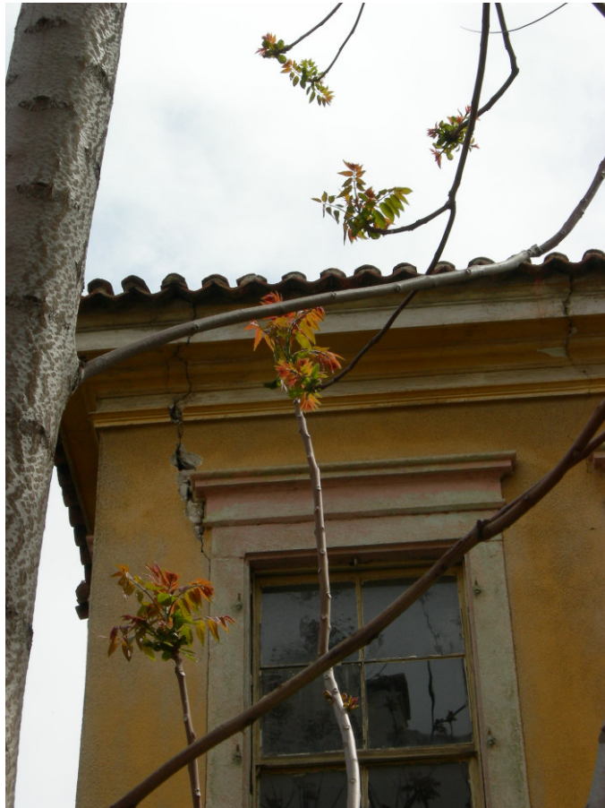
Figure 2.117. The major crack above the window level at the northern corner of western facade.
