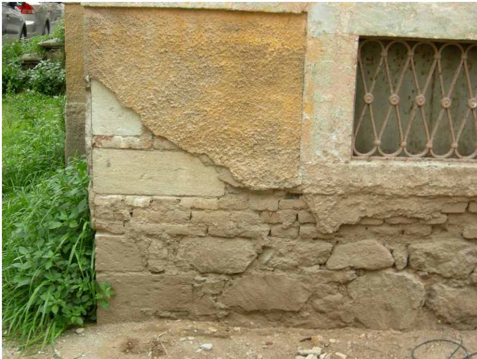
Figure 2.123. The loss of plaster on the bottom part of the exterior walls.
