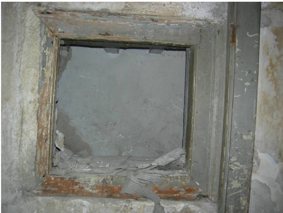
Figure 2.20. The interior window between wet space 2 and the sub-space at the basement floor.
