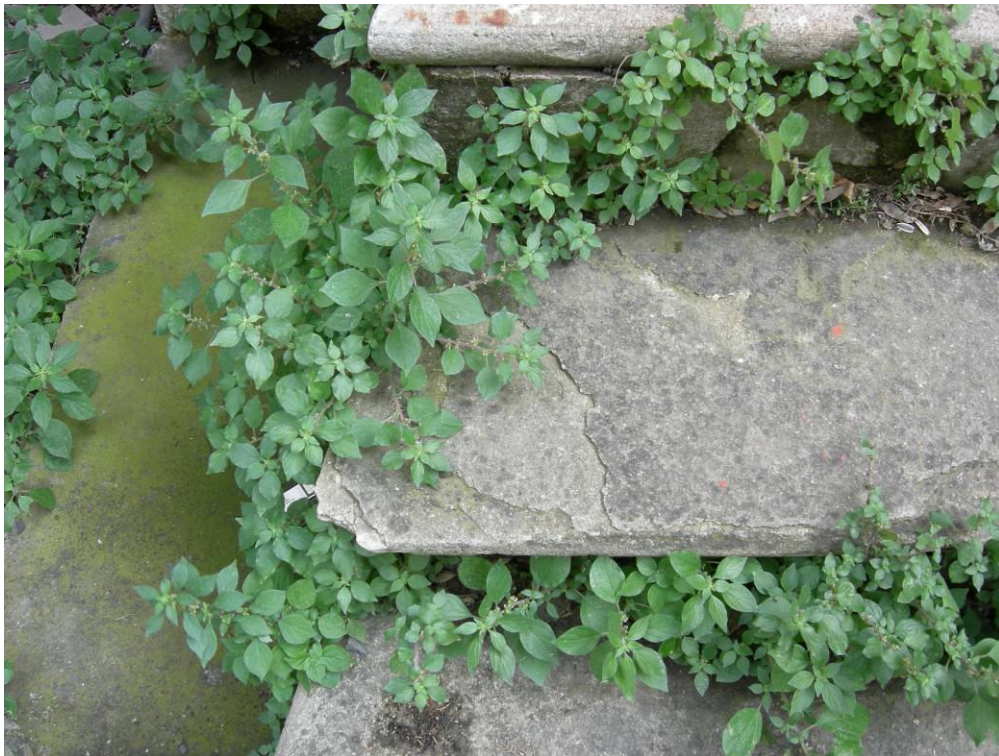
Figure 2.129. Flaking of stone observed on some of the coverings of the terrace.
