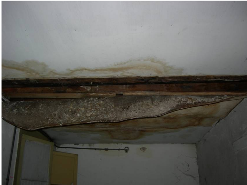
Figure 2.55. The plywood ceiling covering of the storage room at the mezzanine floor.
