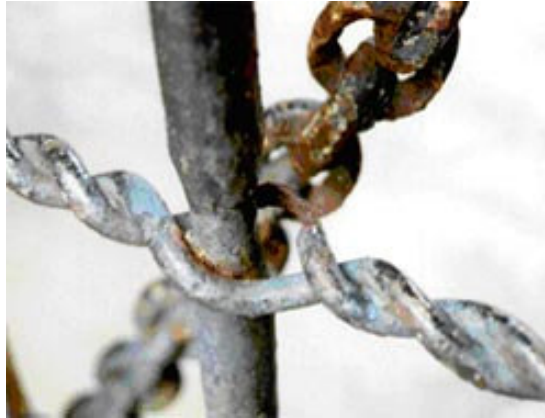
Figure 3.1.9. Fretting corrosion of a fence post and wires. (Source: WEB_10 2007)
