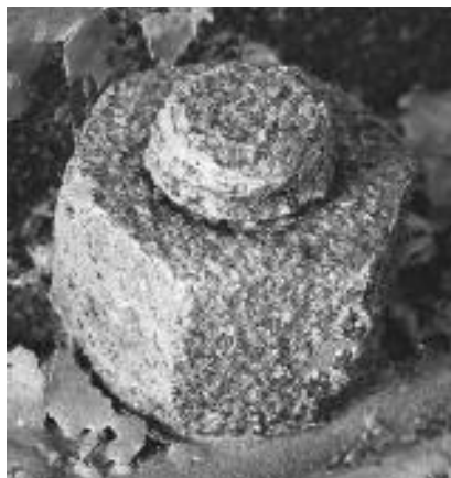
Figure 3.1.6. Rusted metal bolt
