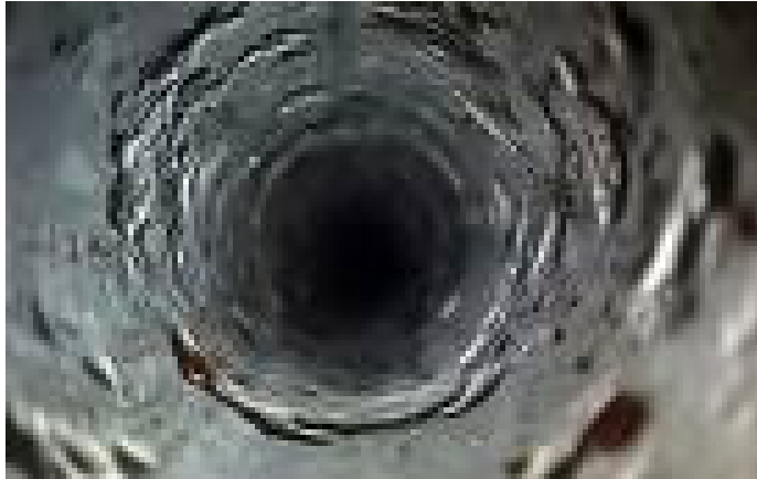
Figure 3.1.2. Deep pitting in exchanger tubes.
