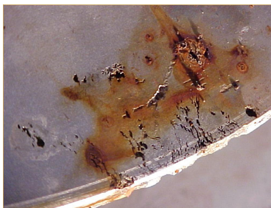
Figure 3.1.10. Stress Corrosion Cracking on Mixer Bearing Support - (CSCC) Chloride Stress Corrosion Cracking, (Source: WEB_11 2007)
