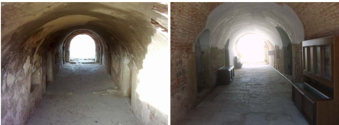
Figure 4.62 Inside of the Namazgah Rampart, main bunker a. before the restoration; b. after the restoration (Source: Ahenk Yılmaz Archive)
