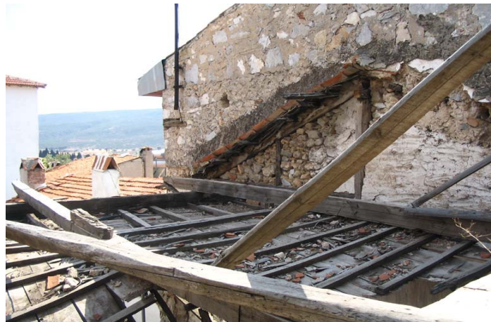
Figure 5.62. Wood plank covering at the bottom of roof which form the ceiling of the first floor (next to Çeşme St. No: 2)
