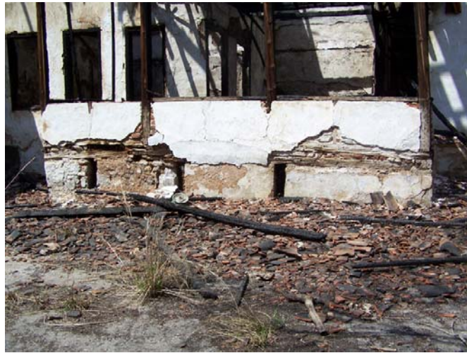
Figure 4.4. Small holes for air circulation on the basement façade wall (Şeyh Cami St. No: 32)
