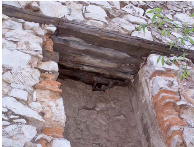
Figure 5.19. Opening of a built-in cupboard formed with wall plates (Konakaltı St. No: 5)
