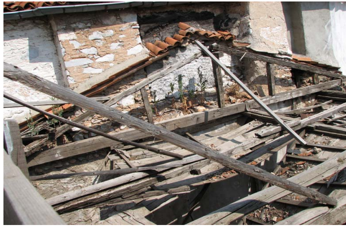
Figure 5.57. Slope of roof is formed with wood trusses, supported by post and studs, placed on ridge purlin and tie beam (next to Çeşme St. No: 2)
