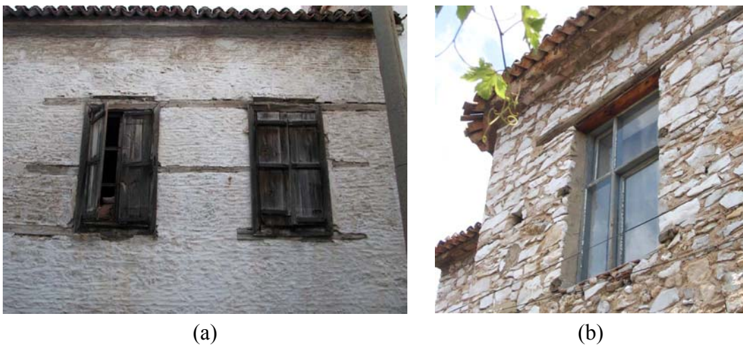
Figure 5.18. Wall plates placed at the mid of opening to fix jambs a. Yayla St. No: 13, b. Camcı St. 2nd dead end No: 36
