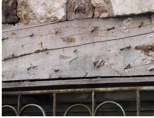
Figure 5.29. Using nails to hold plaster applied on wood elements (Şeyh Cami St. No: 32)
