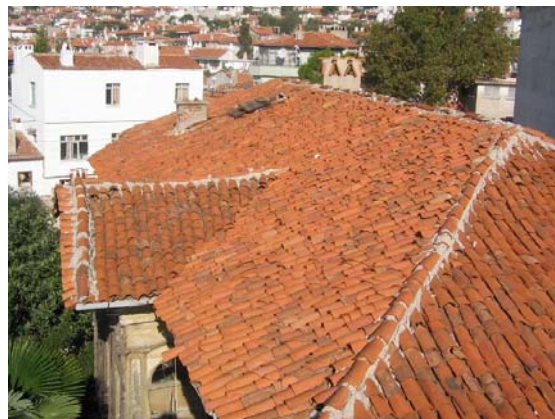
Figure 5.64. Intersection of pitched roof over the triangular pediment of cumba with the hipped roof (Arasta St. No: 9)
