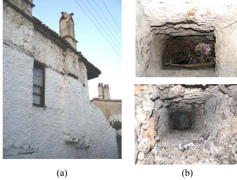
Figure 5.22. a. Protrusion of fireplace in first floor set on big stones placed in the wall (Yayla St. No: 18). Views from the inside of chimney (Şahidi St. No: 26). b. through fireplace, c. through upper part of chimney
