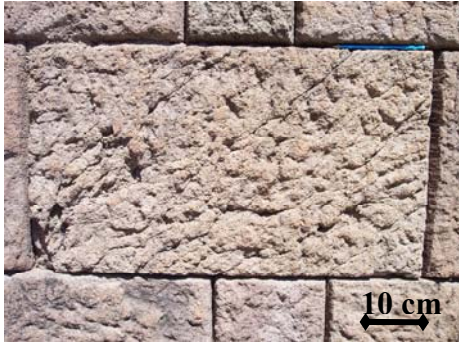
Figure 19. Relief observed on the stone surfaces of Agora
