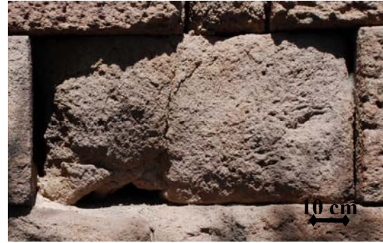
Figure 33. Granular disintegration observed on the stones of Agora
