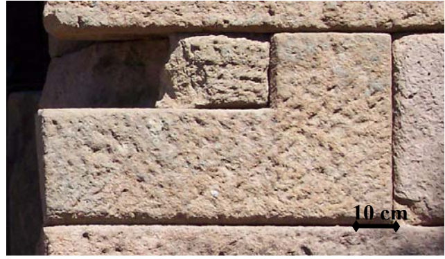
Figure 24. Break out observed on some parts of the building stones of Agora
