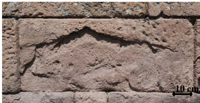
Figure 21. Back weathering observed on the stone surfaces of Agora
