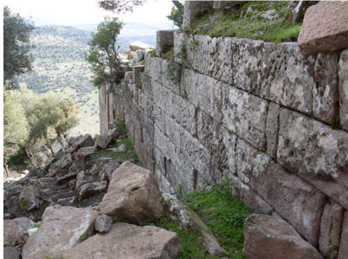
Figure 70. Lichen colonization on the northeast facade of the building
