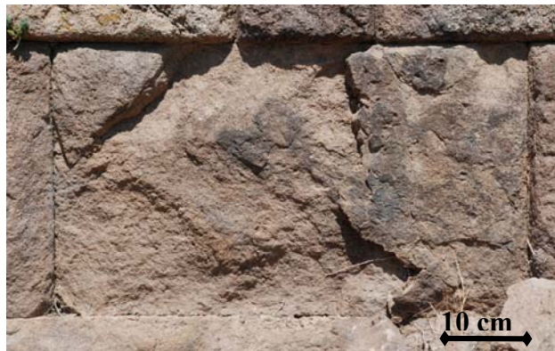
Figure 22. Back weathering observed on the stone surfaces of Agora
