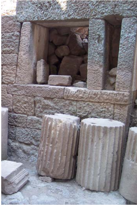
Figure 73. Efflorescence on the surfaces of vertical and horizontal stone blocks defining the entrance to the 7th interior chamber
