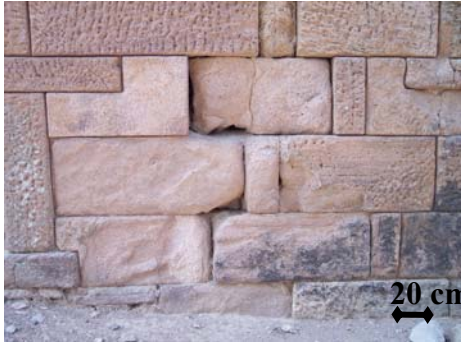
Figure 32. Granular disintegration observed on the stones of Agora
