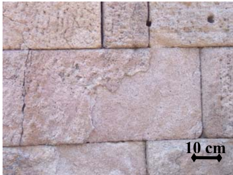
Figure 34. Scaling observed on the stone surfaces of Agora
