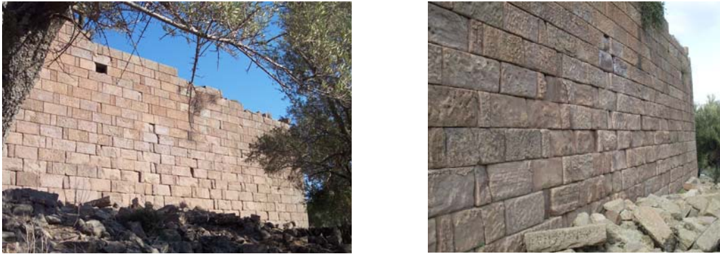
Figure 41. Effect of efflorescence and granular disintegration
