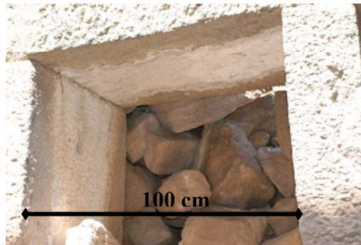
Figure 29. White deposition observed on the lintels of door and window openings of Agora
