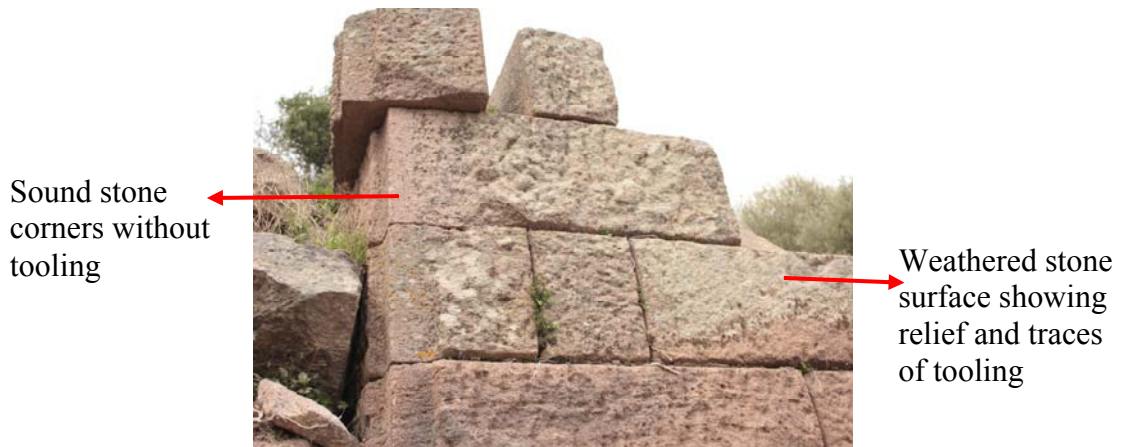
Figure 40. Relief and traces of tooling on stone surfaces and the sound corner parts without tooling at the southeast corner of the building
