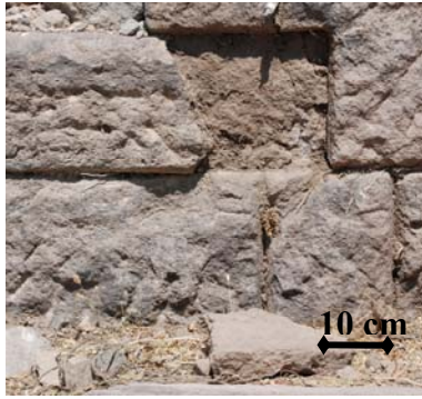
Figure 23. Break out observed on some parts of the building stones of Agora
