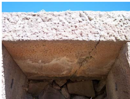
Figure 43. Fissures formed on the lintels of door and window openings
