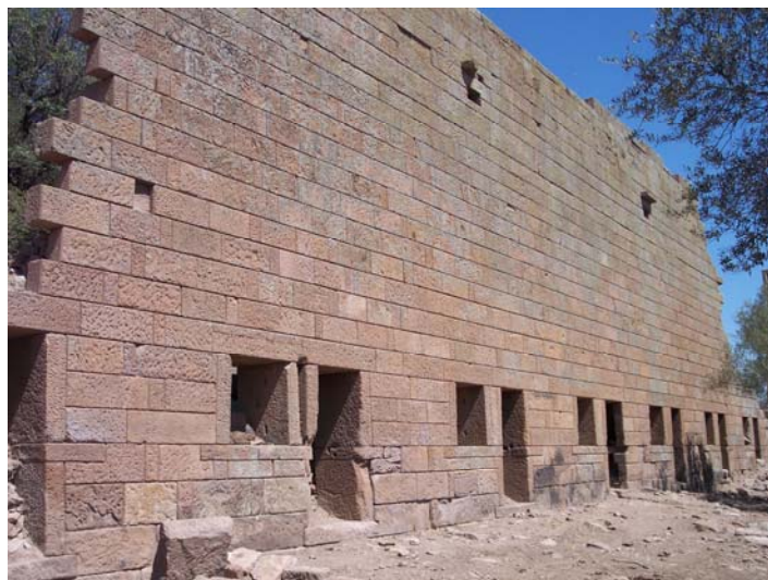
Figure 69. Lichen colonization on the upper parts of the wall
