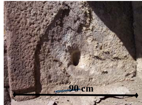
Figure 35. Scaling observed on the stone surfaces of Agora
