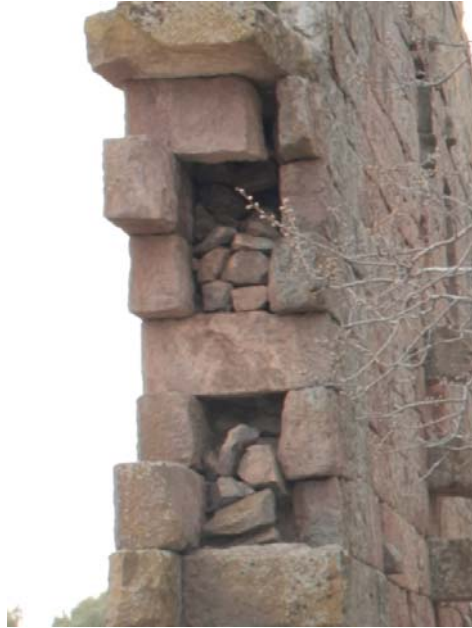
Figure 13. Section of the Southeast wall showing infill material with soil and pebble stone
