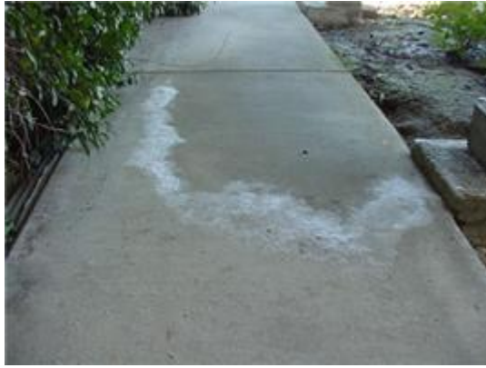
Figure 2.23. Efflorescence of surface [40]
