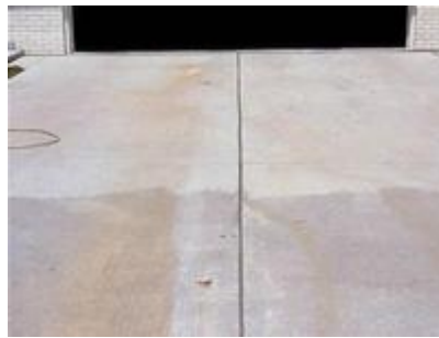
Figure 2.22 Discoloration of concrete [40]
