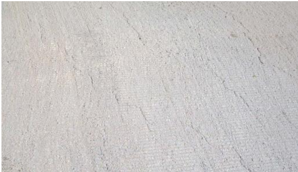
Figure 2.18. Cracking on surface [36]
