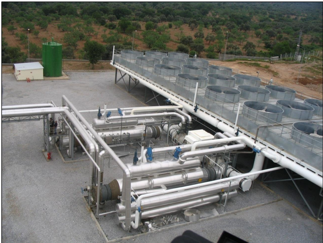
Figure 4.1. General view of DORA-1 GPP
