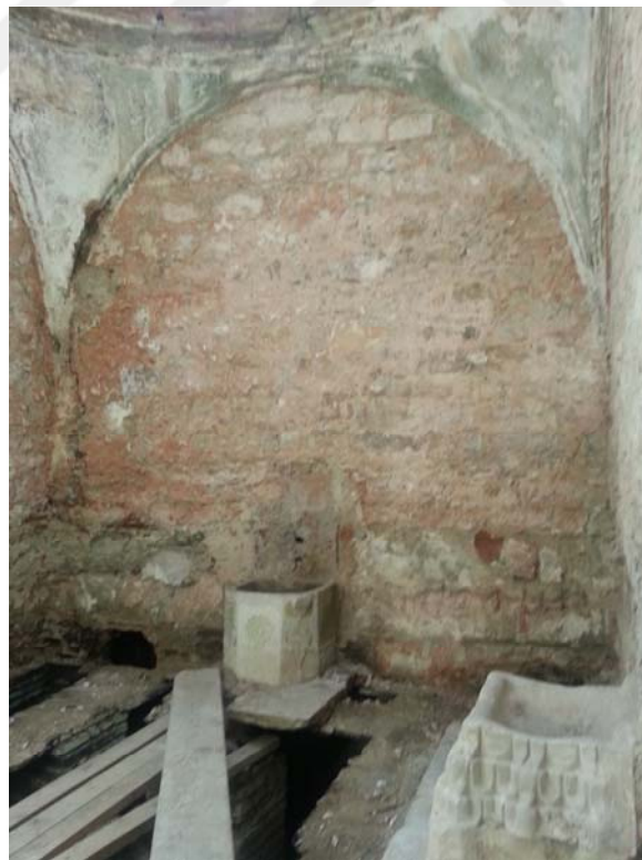
Figure 3.25. Wash basins in the southeast halvet .
