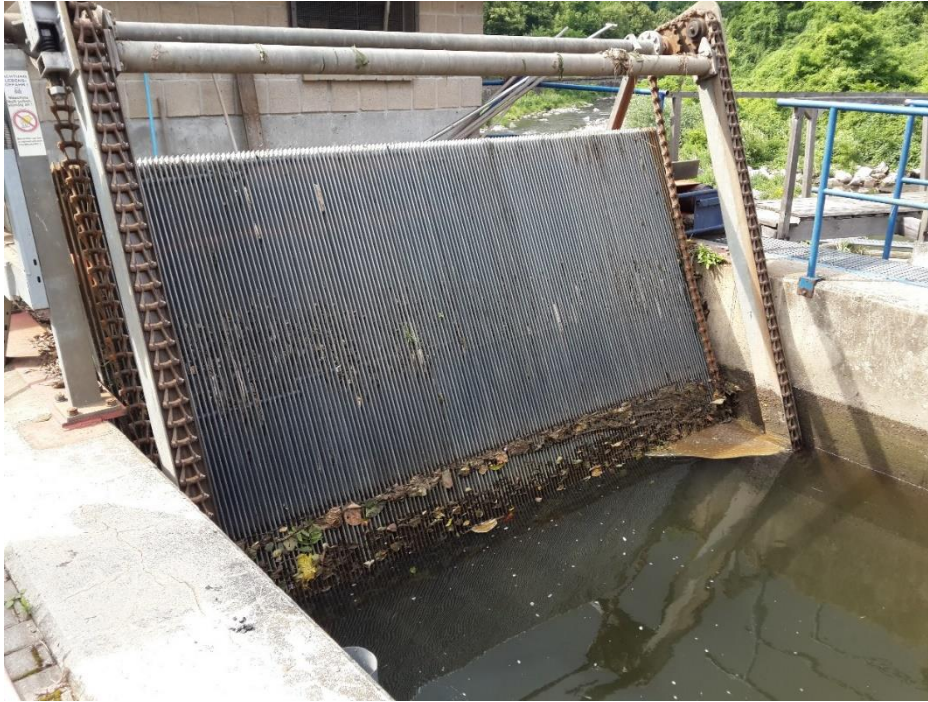
Figure 5.5 : Intake screen in front of the turbines of hydro power plant next to WKA Bienertmühle weir (July, 2014).
