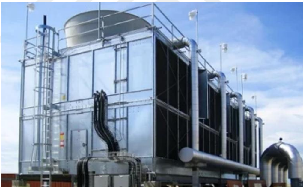
Figure 4.11. Commercial Cooling Tower [65]
