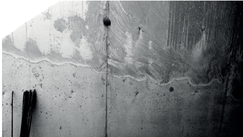
Figure 2.1 Successive casting problems
