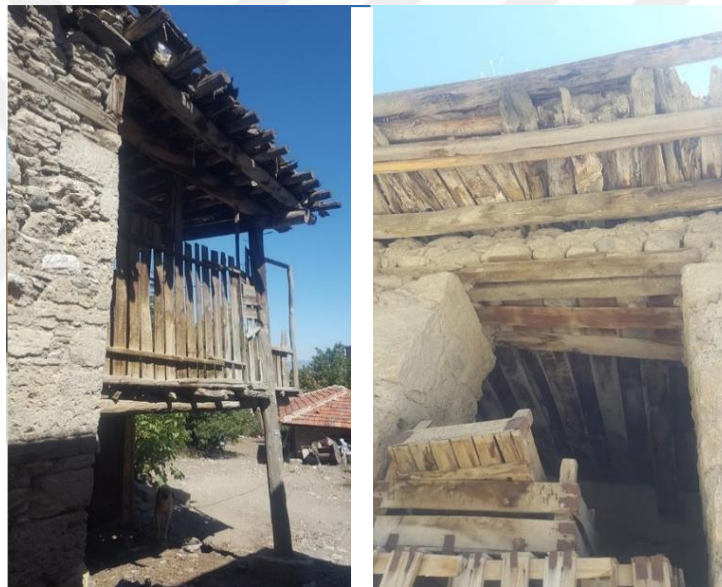
Figure 4. 9. Views of an abandoned house and materials.
