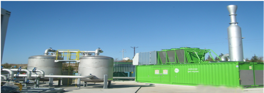
Figure 3.22 : LFGTE plant in Gaziantep (CEV, 2010).
