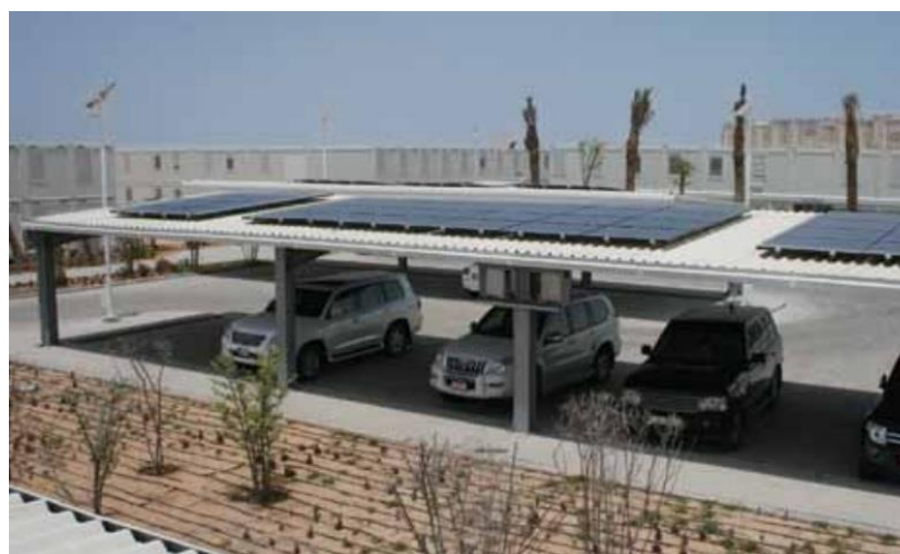
Figure 3.27 : Photovoltaic Parking Shade Structure (Url-7)
