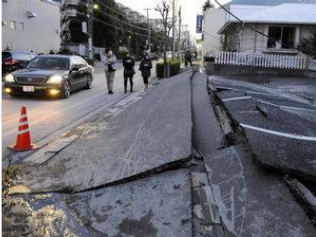
Figure 1.4 : Liquefaction in Urayasu city, outside Tokyo, created an uneven buckling and settling of roads and the surface (Toshifumi Kitamura/AFP/Getty Images).
