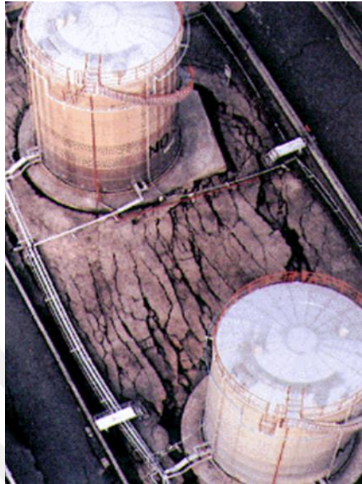
Figure 1.2 : Tanks in the port area. The ground shows signs of massive liquefaction and settlement. The tanks appear to be on pile-supported foundations (The January 17, 1995 Kobe Earthquake an EQE Summary Report).
