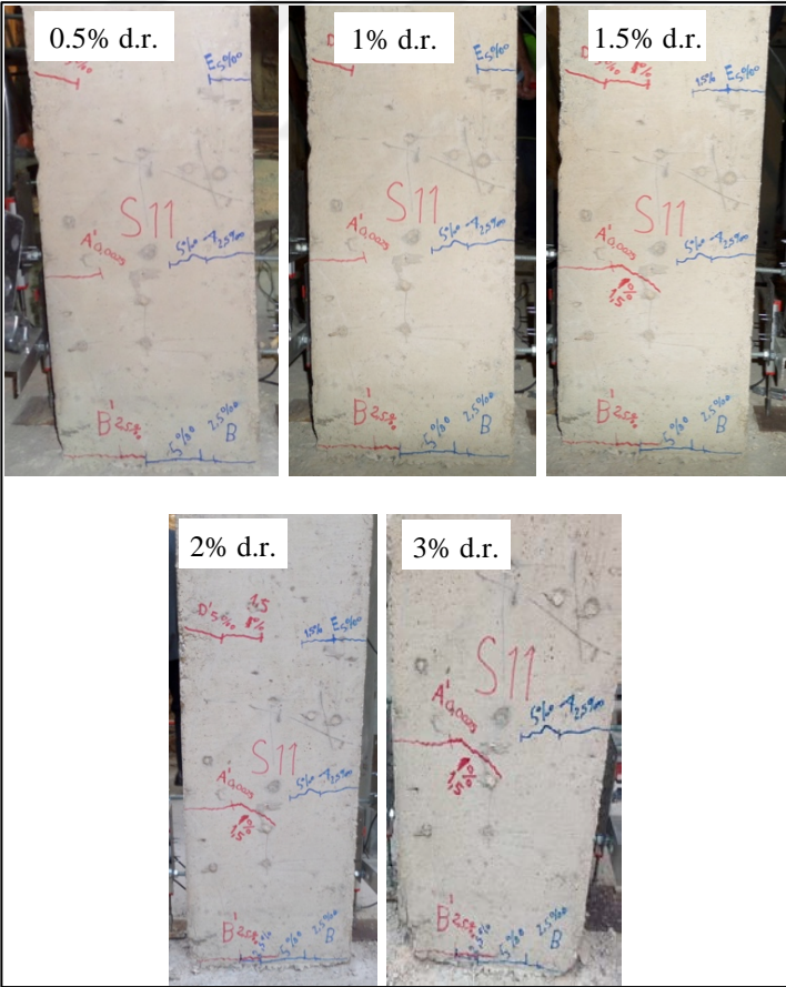
Figure 2.17 : Damage propagation on the 1 st story column S11 of the building TB-2 (Goksu et al. 2015).
