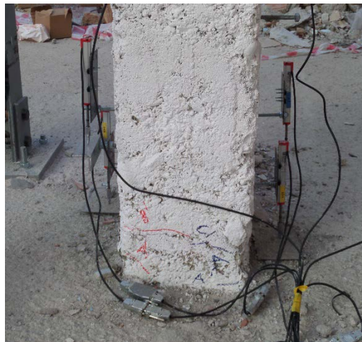
Figure 2.14 : Slight damage on the columns S12 (Comert 2016).
