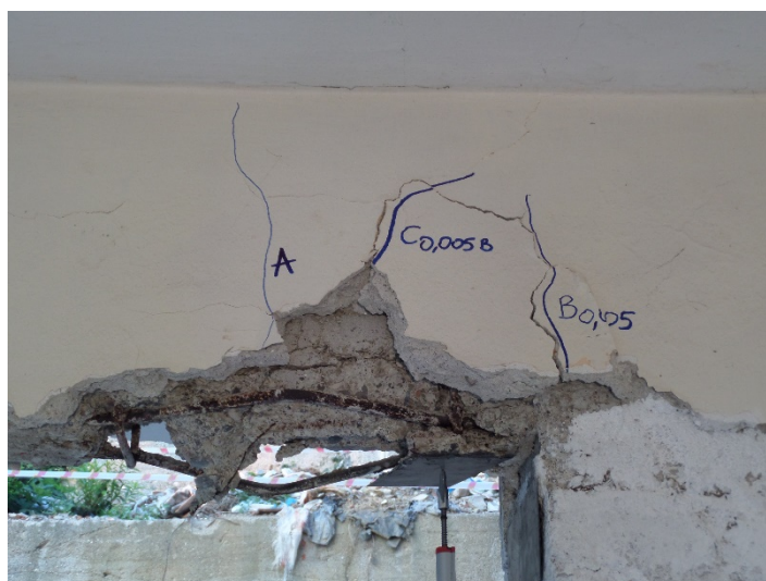
Figure 2.12 : Buckling of bottom longitudinal bars of the beam K12.
