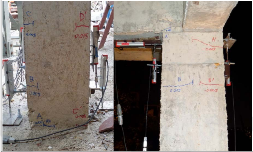
Figure 2.16 : The first observed flexural cracks (a) Column S12 (the 1 st story), (b) Column S14 (the 2 nd story), (Comert 2016).
