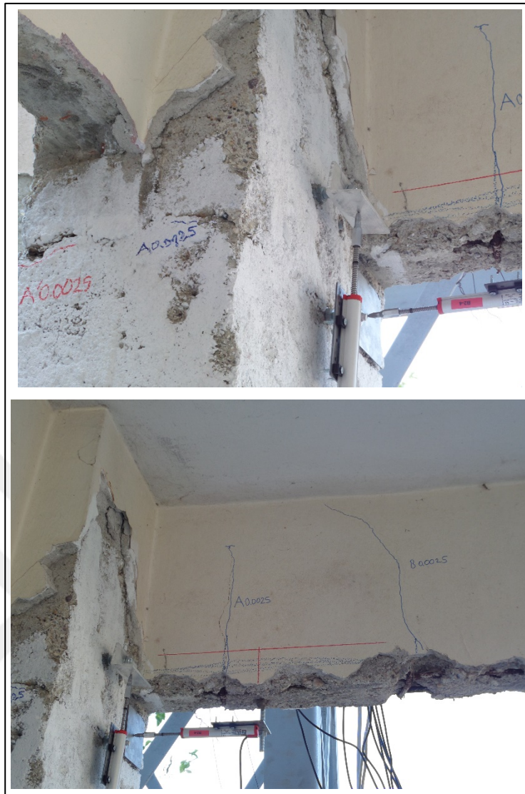
Figure 2.11 : Flexural cracks observed at column S13 and the beam K11 (Comert 2016).
