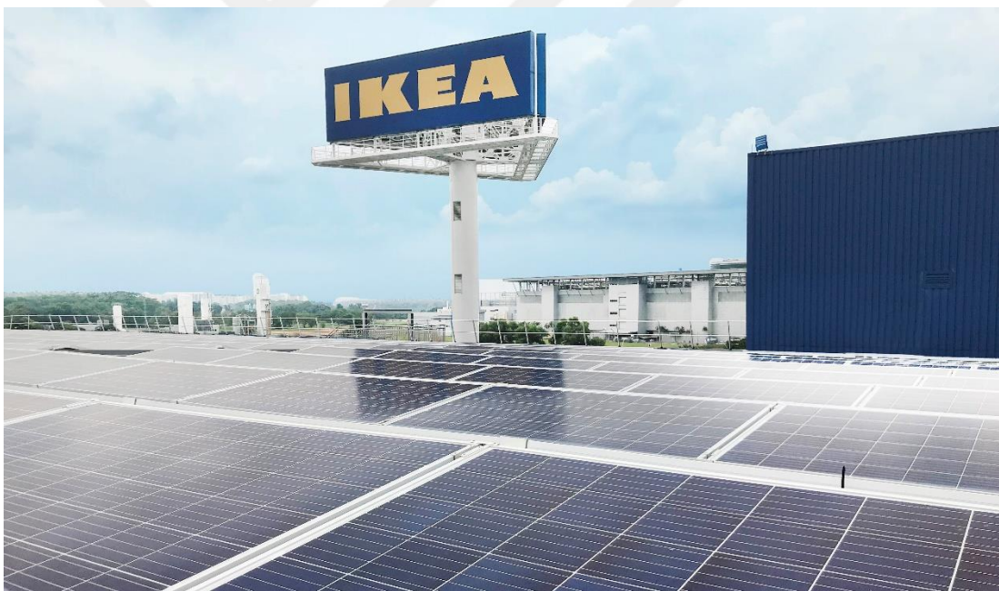
Figure 2.4.1. Solar panels that generates electricity for use in an IKEA store.
