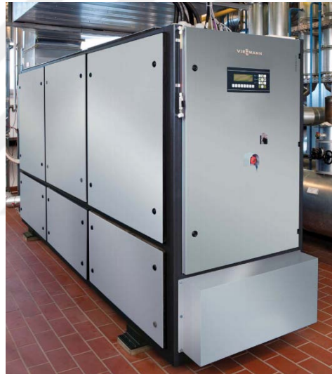
Figure 5.17 : The view of existing cogeneration system in case study building.
