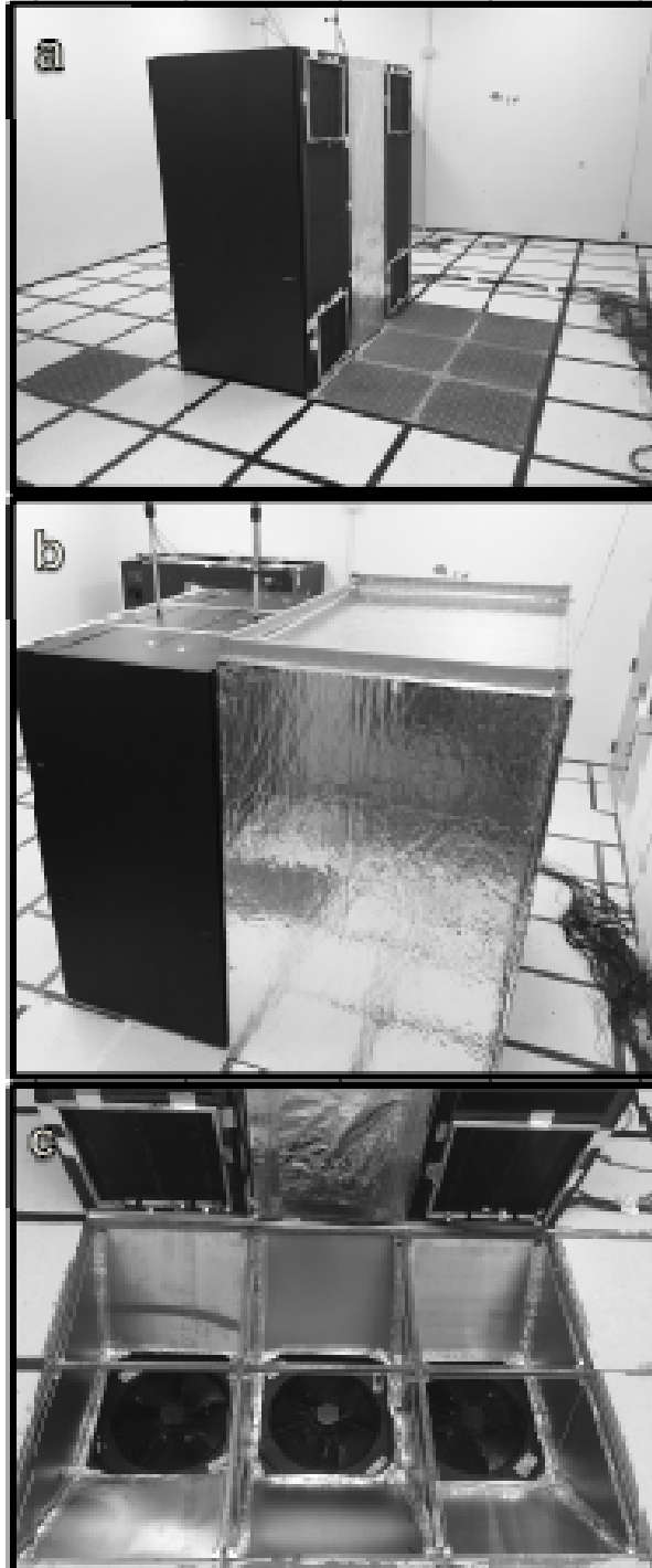
Figure 4.2 : Pictures of GDCRL (a) thermocouple frames, (b) portable cold aisle containment, and (c) installed fans below the perforated tiles in CA .
