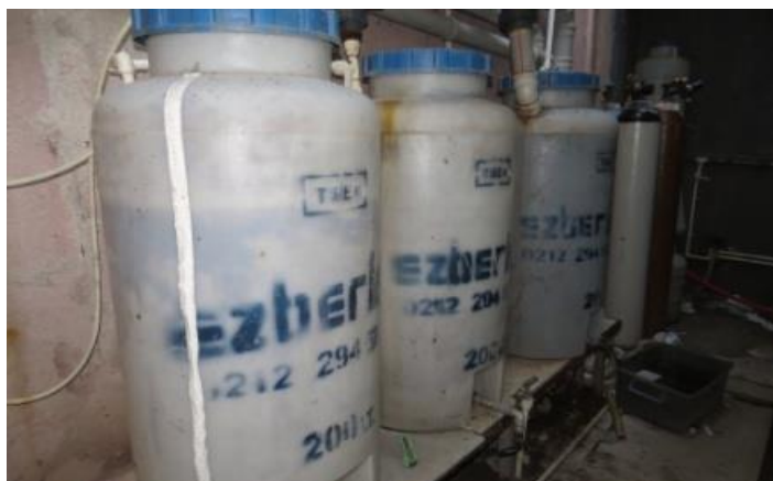
Figure 4.2: Urine collection tanks.
