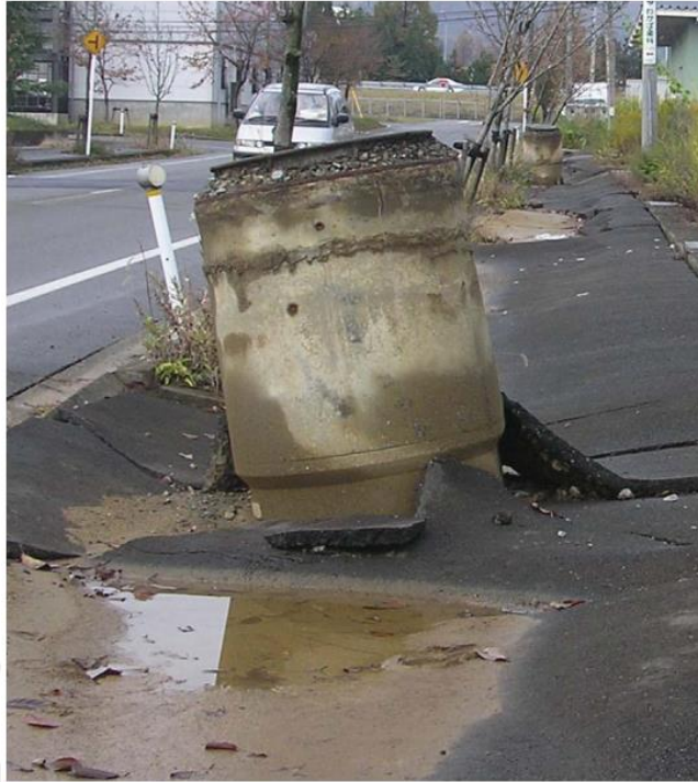
Figure 2.1 : Vertical uplift of manhole and densified surrounded soil.
