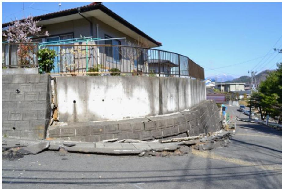
Figure 2.4 : Heaving of soil under retaining wall during Tohoku Pacific Earthquake 2011 (Tokimatsu et al, 2012).
