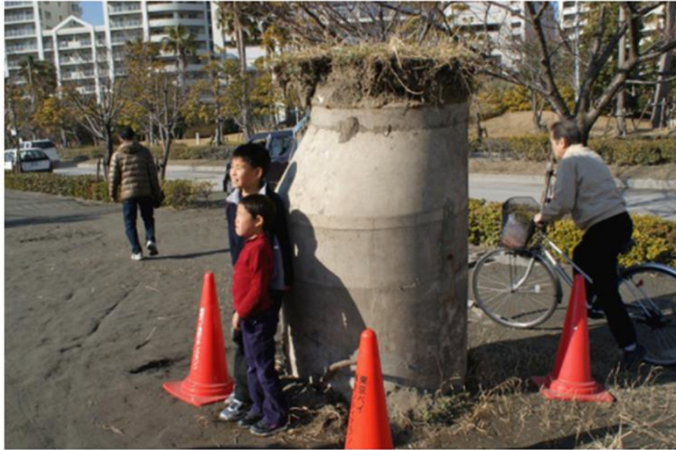
Figure 2.3 : Uplift of manhole during Tohoku Pacific Earthquake 2011 (Tokimatsu et al, 2012).
