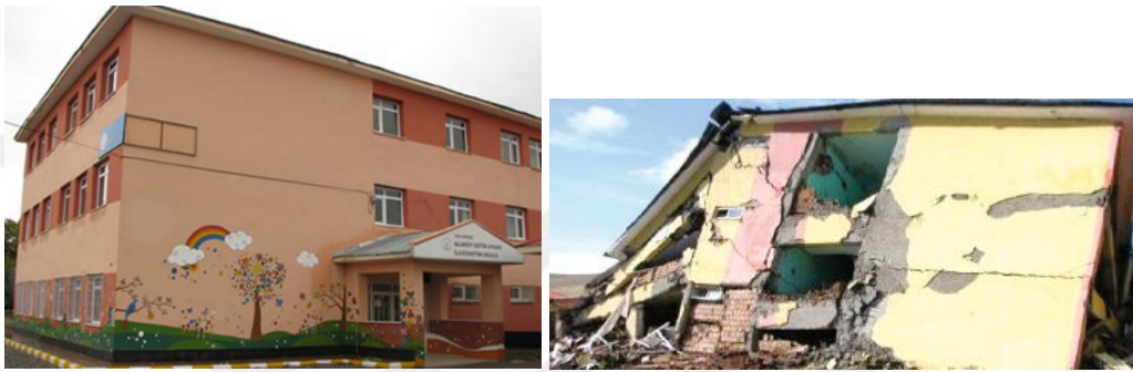
Figure 1.4 : Elementary school buildings of same design. Left: Construction conforming to the original design (EEDMI report). Right: Collapse due to missing shear walls (Yazgan et. al, 2016).
