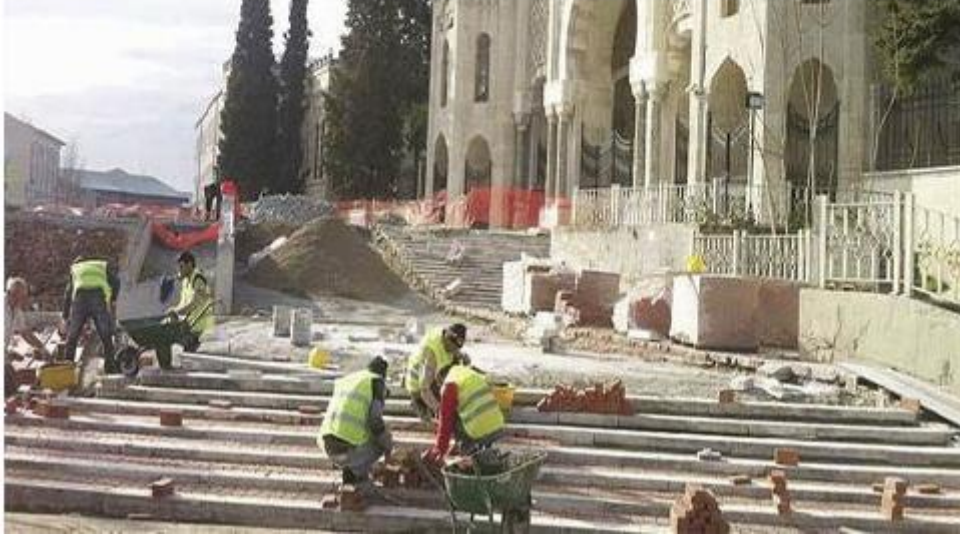
Figure 5.30. Removal of the marble stairs in front of the İstanbul University (Source : http://www.yapi.com.tr/haberler/beyazit-meydanina-mermer-merdivenler-yerine-tugla_128920.html )
