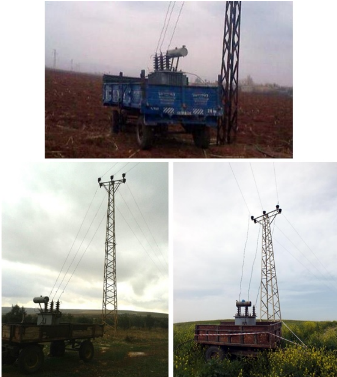
Figure 3.6: Mobile Transformers Used for Agricultural Irrigation Illegally
