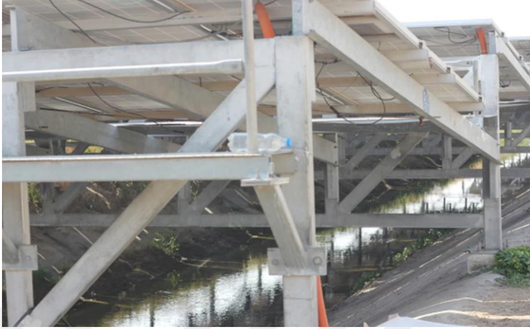
Şekil 3.36 Kanal Suyu Üzerinde Paneller ( http://www.indiaspend.com/cover-story/why-indias-canals-could-help-fast-forward-its-solar-energy-plans-61816 ).
