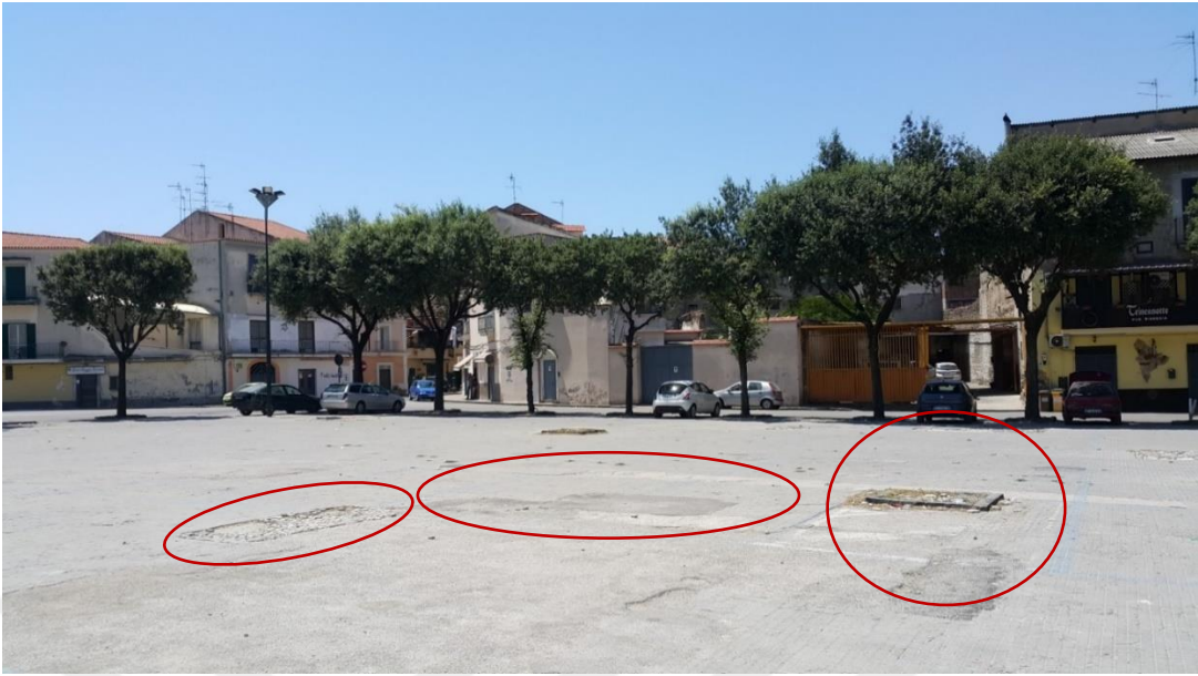
Figure 27.1. Floor Deterioration-2 / Modified Asphalt Operation. (Demirci, Didem,12.06.2017)
