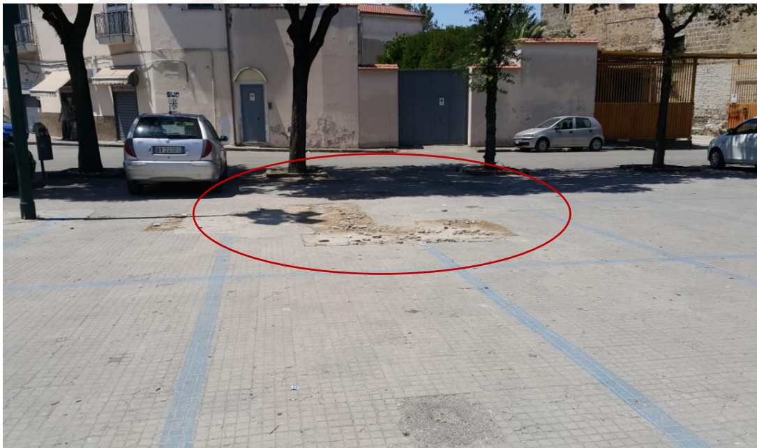
Figure 26. Floor Deterioration/ Fracture and Breakage. (Demirci, Didem,12.06.2017)
