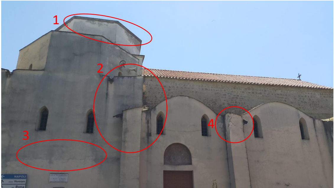
Figure 18.4 North Side Facade of Church of Santa Maria in Piazza Dome Part Corruption-2 (Demirci, Didem,12.06.2017)
