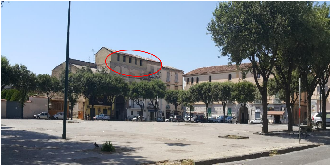
Figure 30.3. Facade Corruption depend on Squalidity & 0 – 1,5 cm Plaster Deformations and affusion. (Demirci, Didem,12.06.2017)
