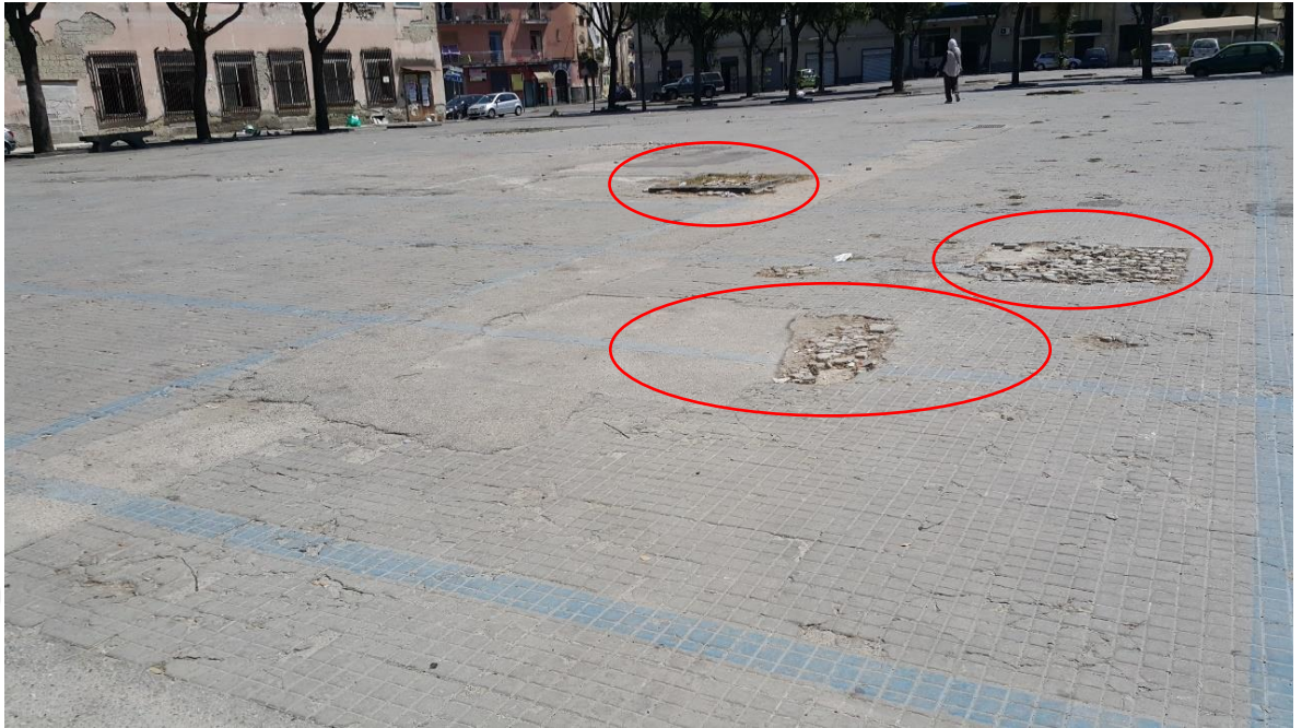
Figure 28. Floor Deterioration-4/ Dismantled Afforestation Damage
