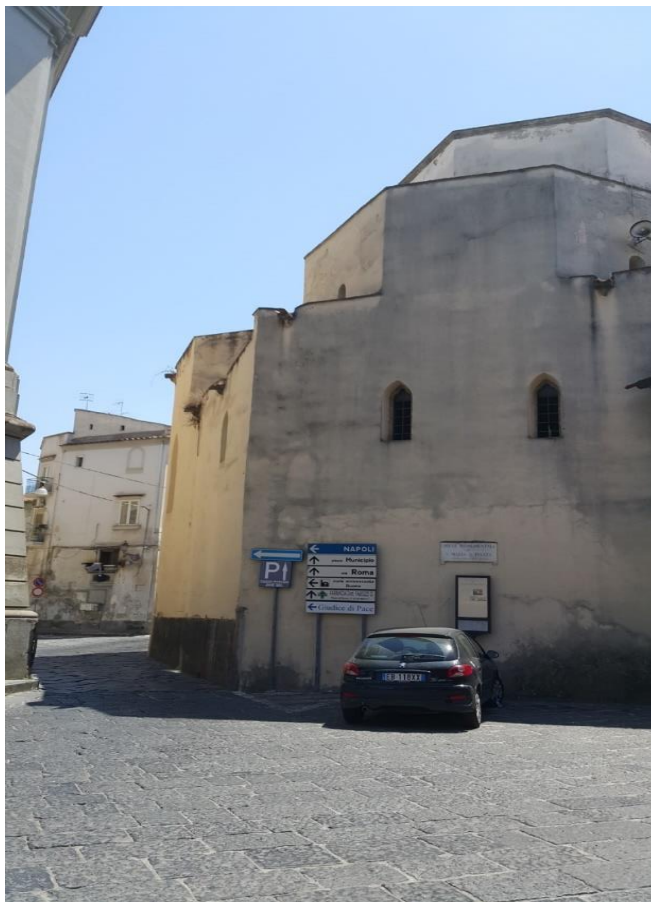
Figure 18.3. North Side Facade of Church of Santa Maria in Piazza Dome Part Corruption-1 (Demirci, Didem,12.06.2017)
