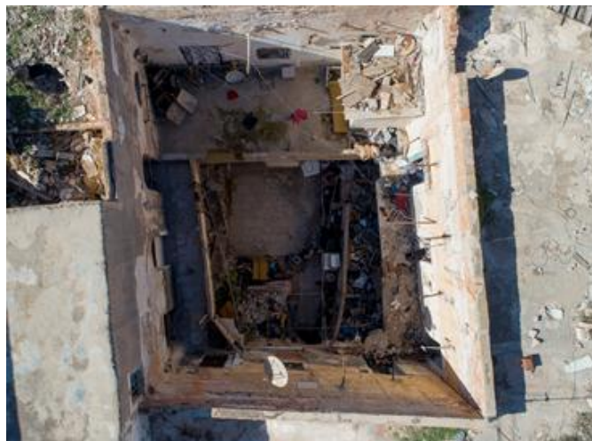
Figure 7.82 Dust and Waste Accumulation
