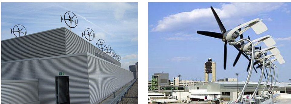
Figure 3.63. Building mounted wind turbine URL[59,60]
