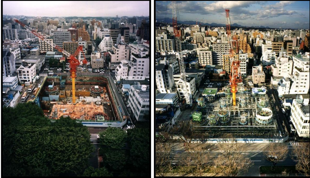
Figure 258: During the construction process of Sendai Mediatheque, positioning and assembling the tubes.
