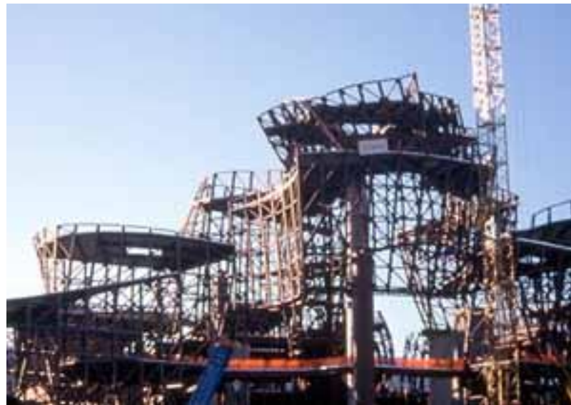
Figure 200: The real structure of the main form indicating the curved steel bars and the wireframe system.
