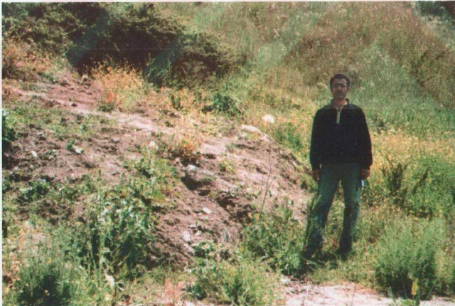
Figure 28: The toe part of the soil flow in the western part of Gürpınar.
