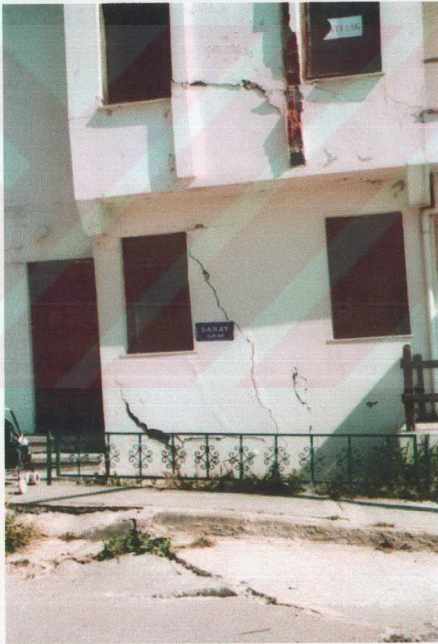
Figure 31: Abandoned and damaged building due to expansion and contraction of the clayey soil in the southern part of Gürpınar.
