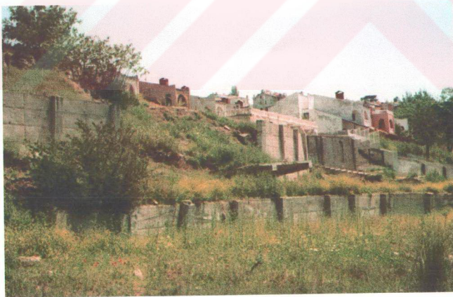
Figure 45: Retaining walls were built incorrectly
