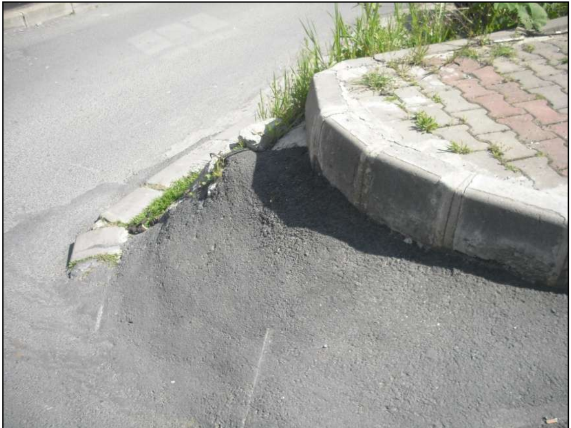
Figure 31. A sample of a dangerous ramp in the study area
