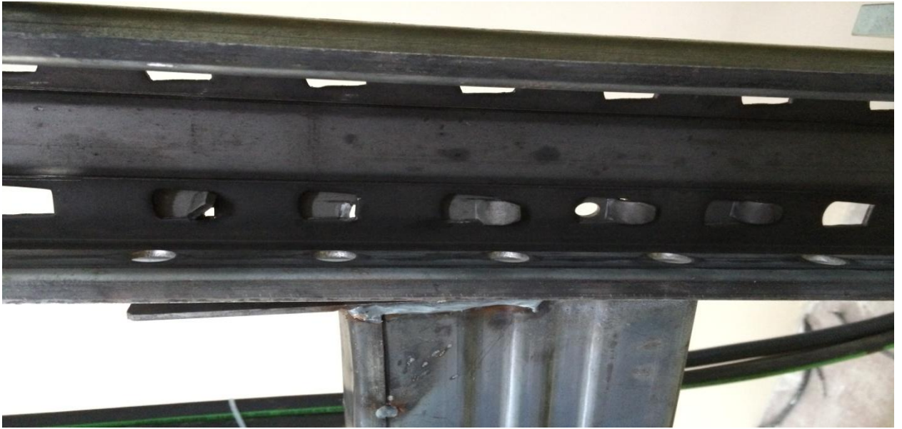
Failed loading joint.
