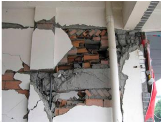
(c) Shear damage to short column and short beam
