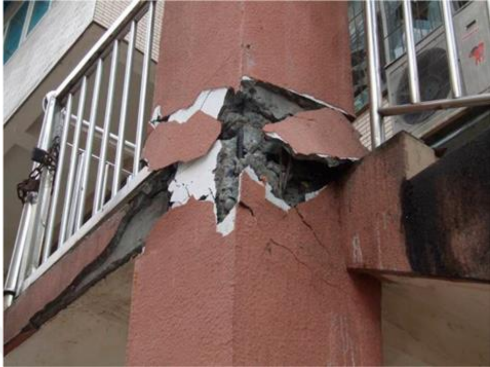
Figure 1.2 Damage on the column due to interaction with staircase (Li and Mosalam, 2013)
