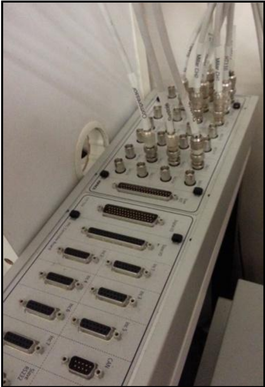
Figure 3.39: dSPACE connections of pressure transducers, flow meter and check valves
