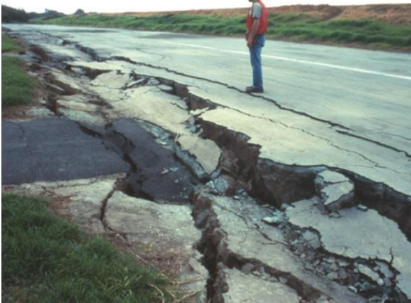
Şekil 1.10. Loma Prieta, California, ABD, foto: Steve Ellen, U.S. Geological Survey (URL-2)
