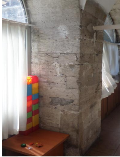
Figure 5.42: Damage of Pillars (B8)
