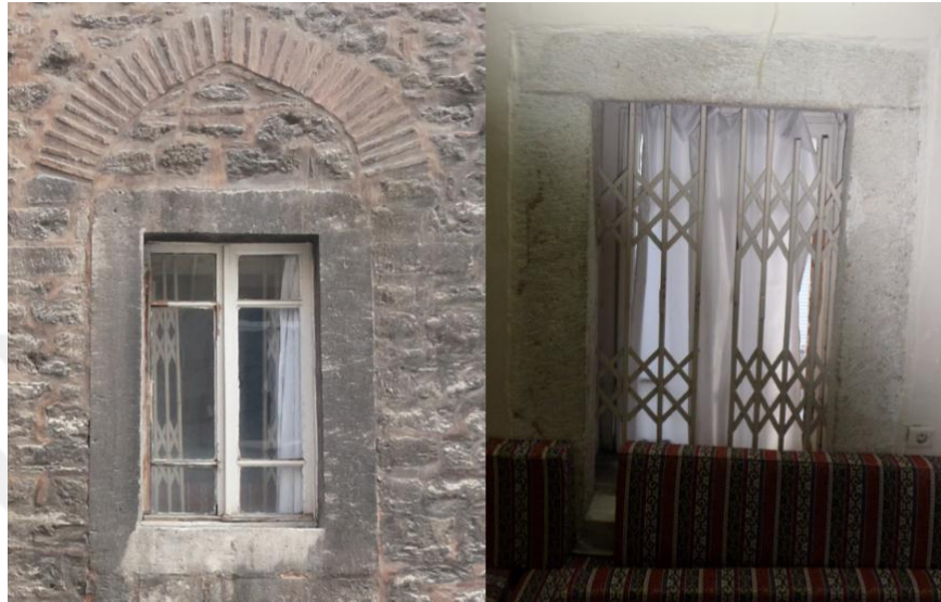
Figure 5.30: Damage of Window (E10E11C10C11) 1. Exterior Face of Window 2. Interior Face of Window
