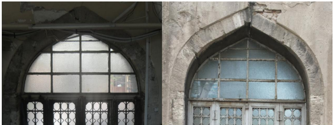
Figure 5.16: Damage of Arch of main entrance (C8C10D8D10) 1. Interior Face of Arch 2. Exterior Face of Arch
