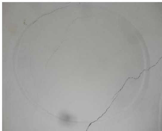
Figure 3.19: Damage of Dome Semiz Madrasa Istanbul
