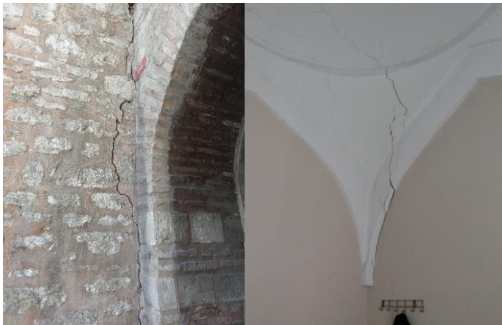
Figure 5.32: Damage of Wall (G8H8) 1. Exterior Face of Wall 2. Interior Face of Wall
