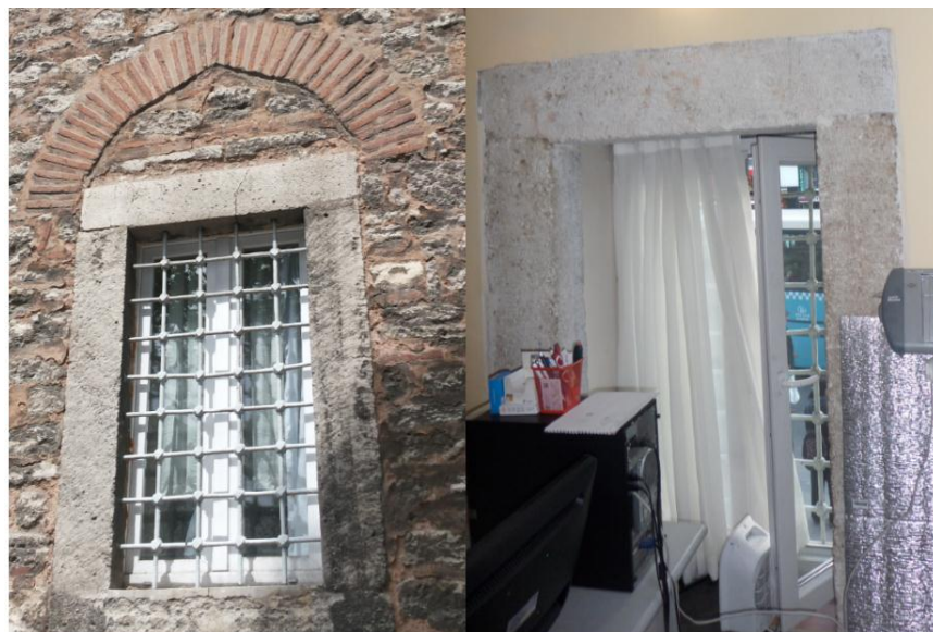
Figure 5.29: Damage of Window (G8G9H8H9) 1. Exterior Face of Window 2. Interior Face of Window
