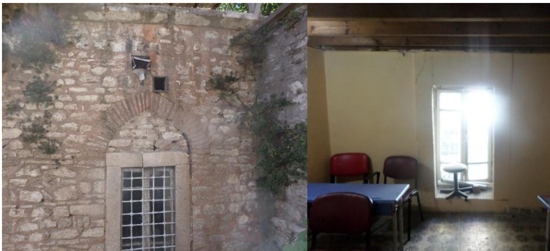
Figure 5.36: Damage of wall (A1B1) 1. Exterior Face of wall 2. Interior Face of Wall
