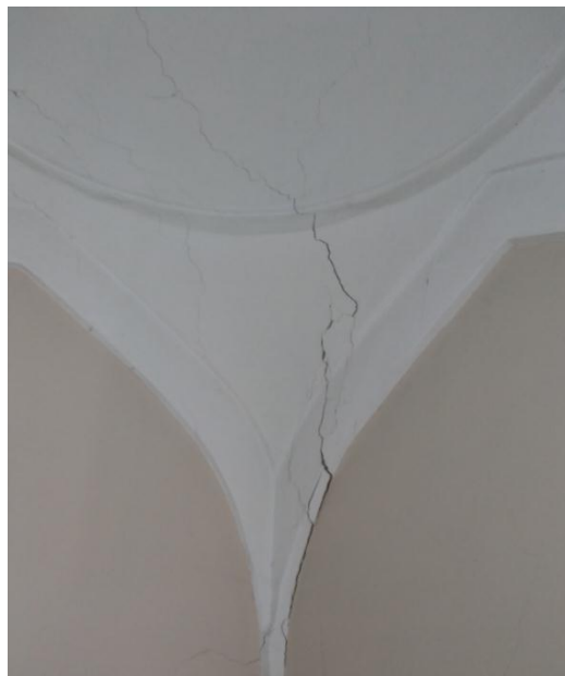
Figure 5.20: Damage of Pendentive of Room (H8H9G8G9)
