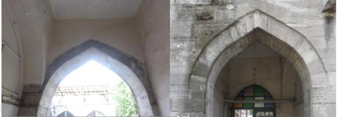
Figure 5.15: Damage of Arch (E7E8G7G8) 1. Interior Face of Arch 2. Exterior Face of Arch
