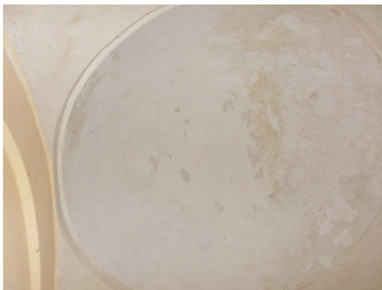
Figure 5.4: Damage of Dome (E1E2G1G2)
