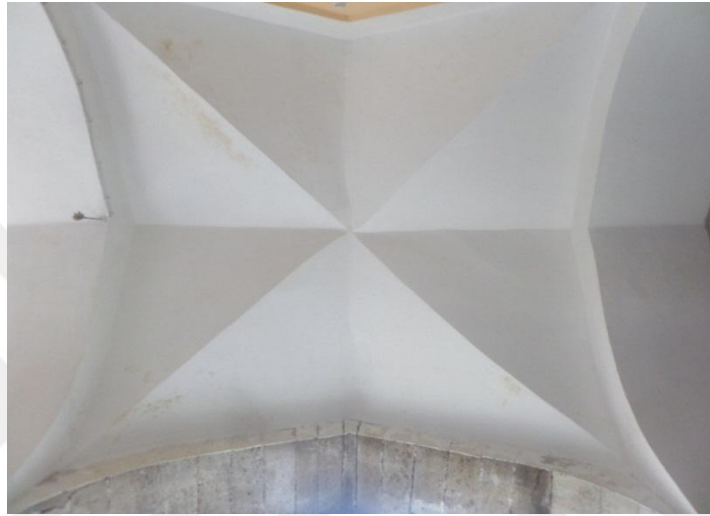
Figure 5.11: Damage of Cross Vault (E9E10F9F10)
