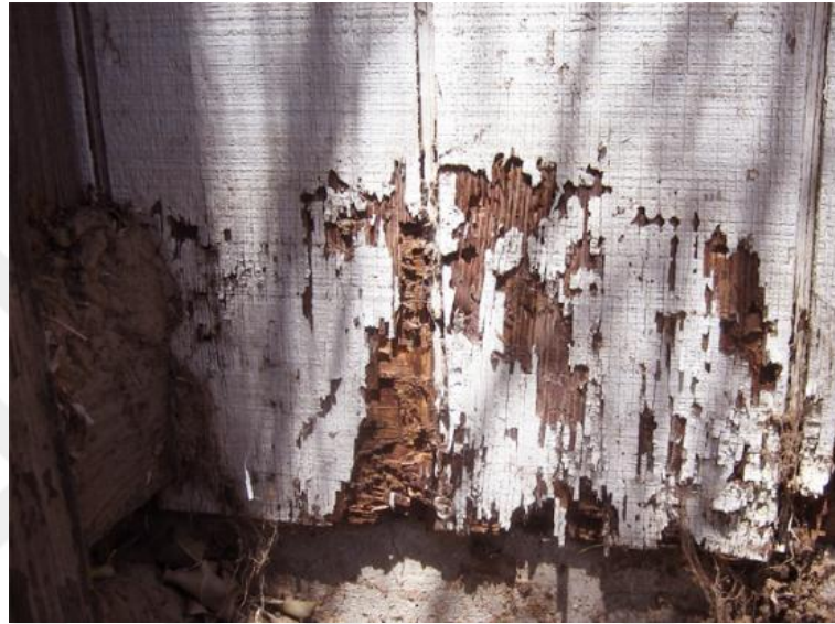
Figure 3.3: Insect Damage (Termites) on Wood
