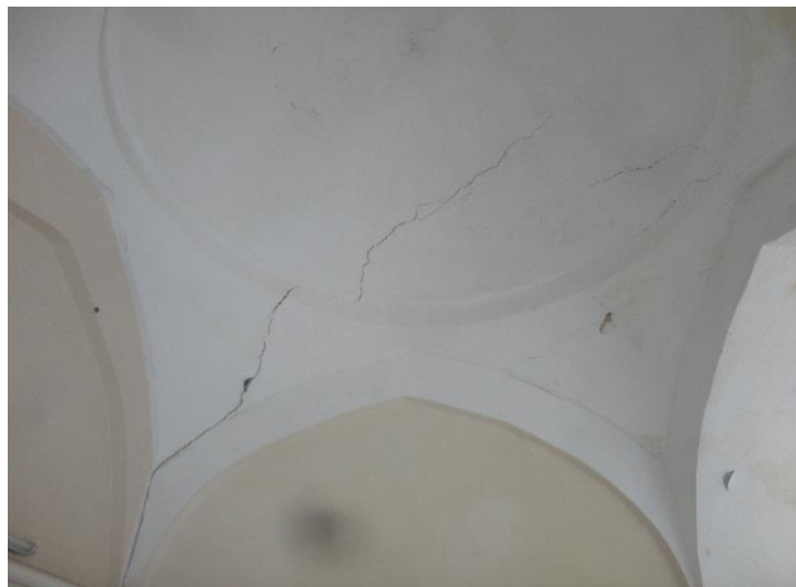
Figure 5.18: Damage of Pendentive (A2A3B2B3)
