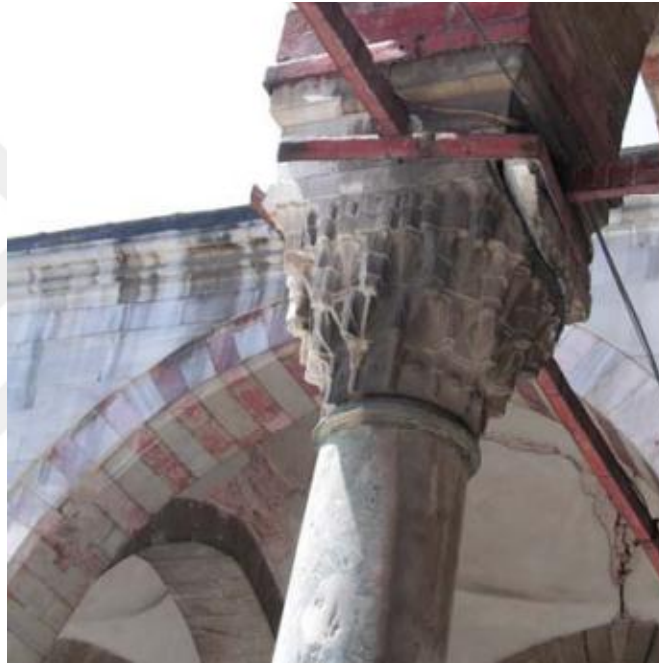
Figure 3.11: Damage of the Metal Braces on Column
