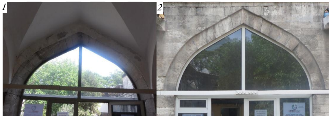
Figure 5.13: Damage of Arch (E8E10D8D10) 1. Interior Face of Arch 2. Exterior Face of Arch
