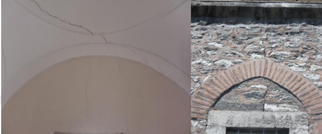
Figure 5.33: Damage of wall (H10H11) 1. Exterior Face of Wall 2. Interior Face of Wall
