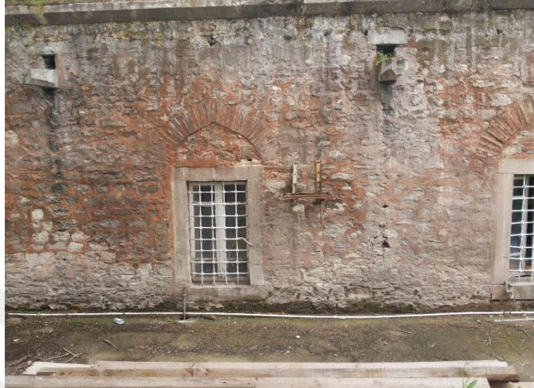
Figure 5.39: Damage of Wall (D1F1)
