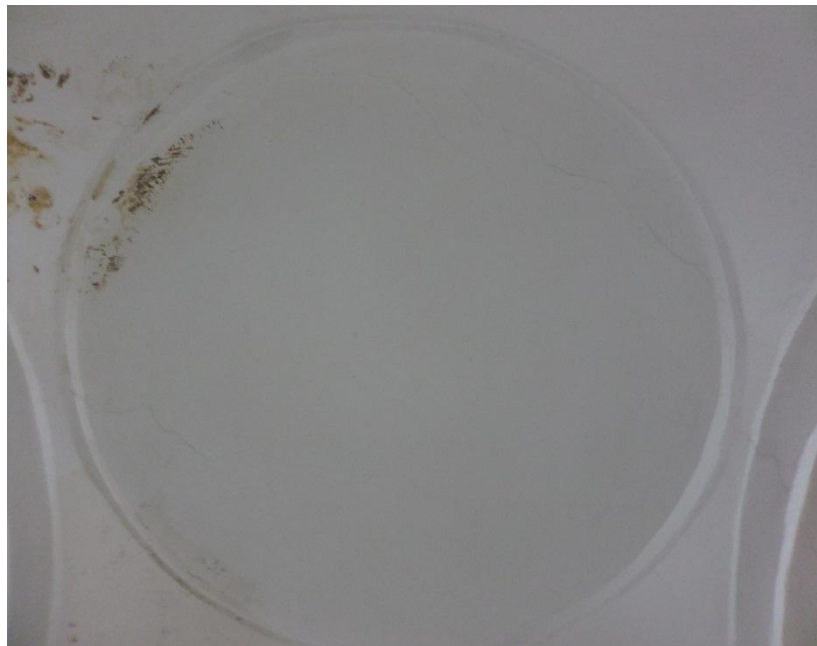
Figure 5.10: Damage of Dome (C10C11B10B11)
