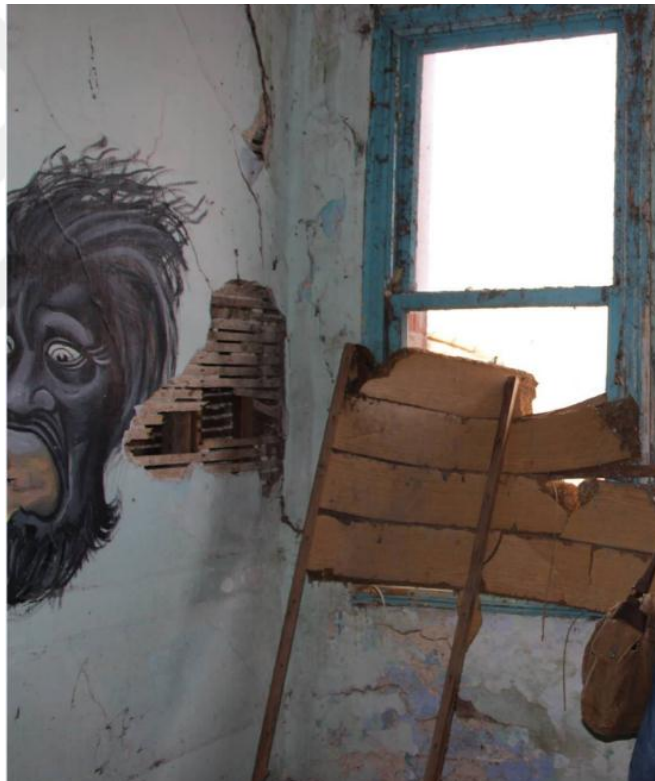
Figure 3.8: Damage in a Building Used as a Homeless Shelter
