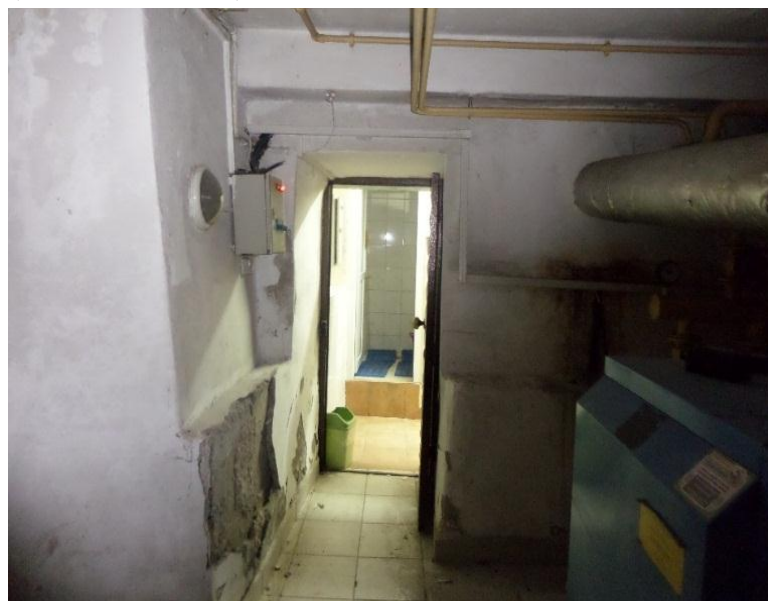
Figure 5.40: Damage of Basement Room (A10A11B10B11)
