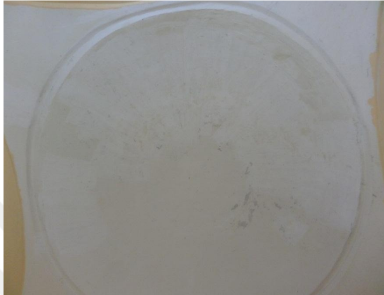
Figure 5.5: Damage of Dome (G1G2H1H2)
