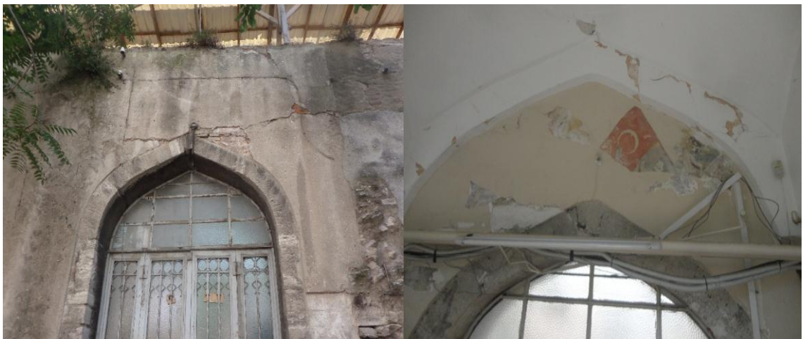
Figure 5.38: Damage of wall (A6A7) 1. Exterior Face of wall 2. Interior Face of Wall
