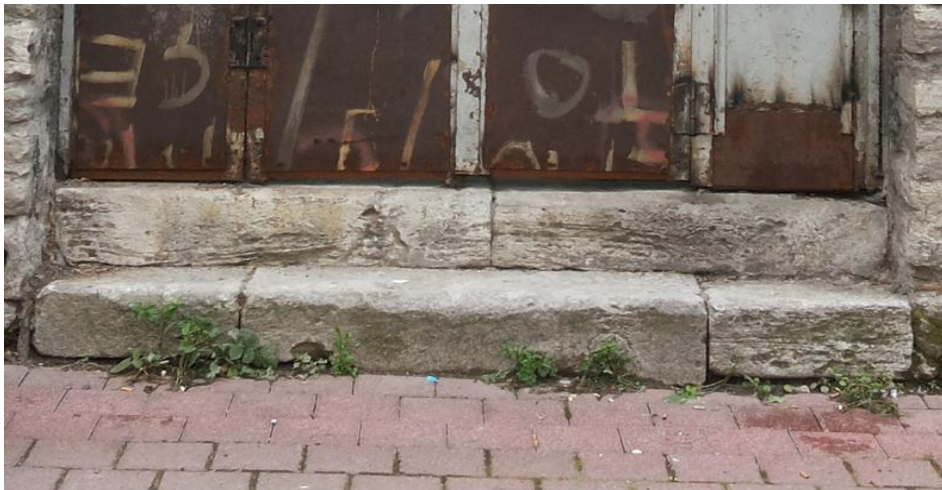
Figure 5.28: the Damage of Stairs of the Old Entrance (A6A7B6B7)
