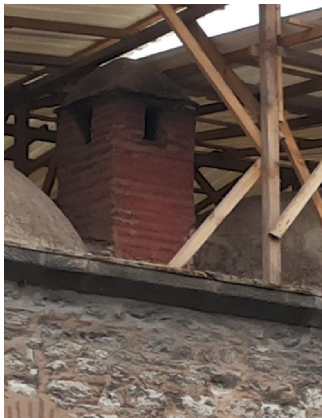
Figure 5.26: Damage of Chimney's Stacks
