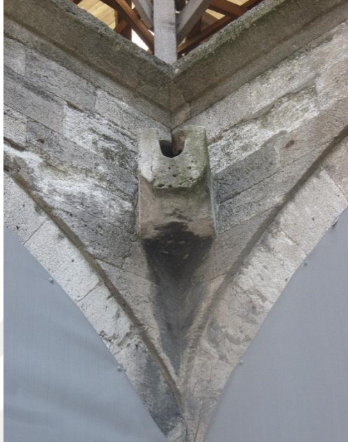
Figure 5.25: Damage of Rain Gutter (G2G3F2F3)
