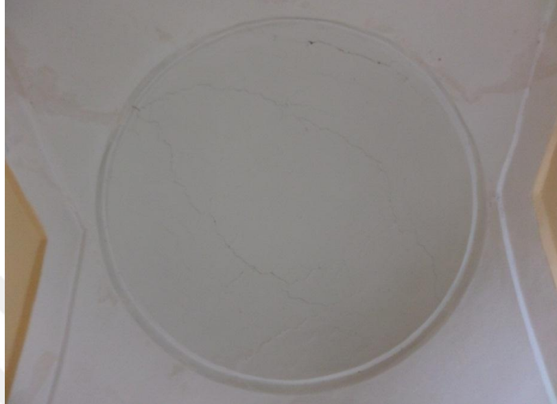
Figure 5.7: Damage of Dome (H8H9G8G9)
