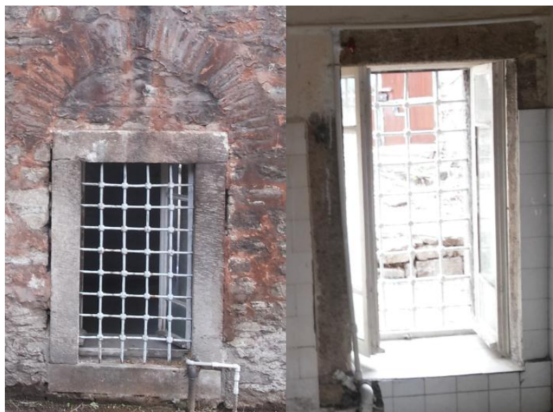
Figure 5.31: Damage of Window (G1G2E1E2) 1. Exterior Face of Window 2. Interior Face of Window
