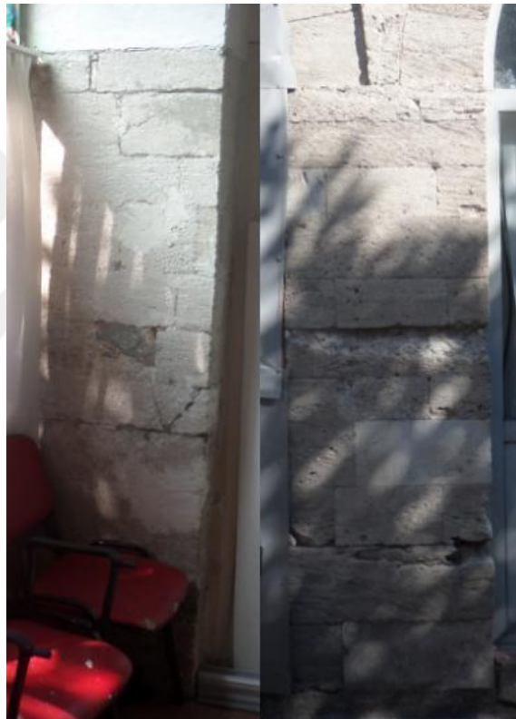
Figure 5.41: Damage of Pillars (B4)
