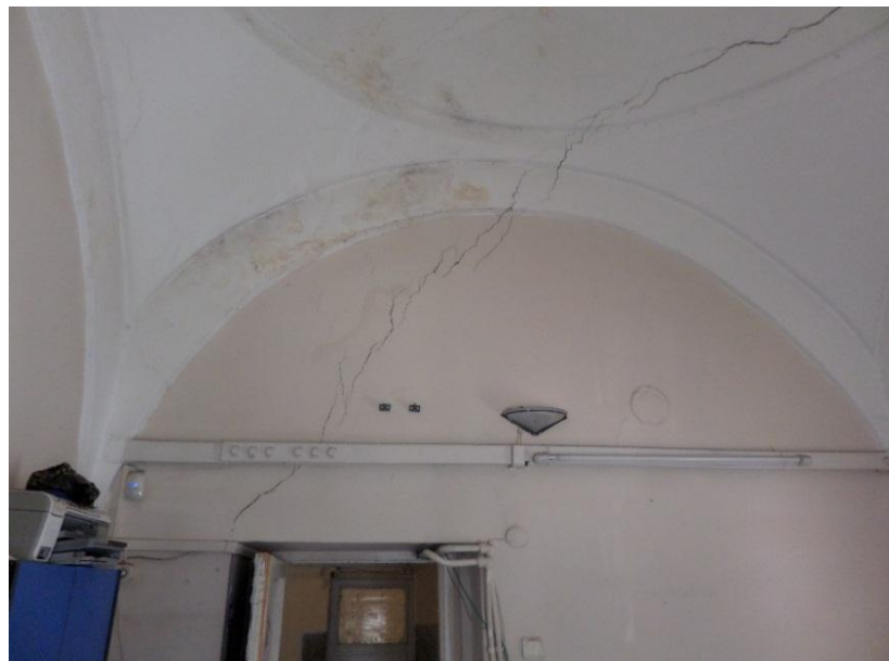
Figure 5.34: Damage of Wall (H10G10)
