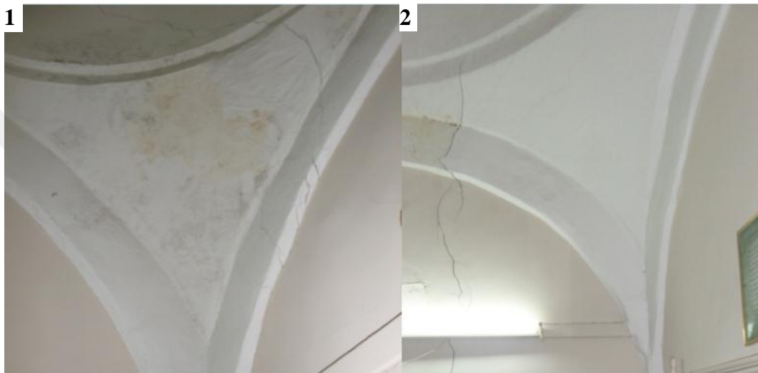
Figure 5.17: Damage of Pendentive (G10G11E10E11)
