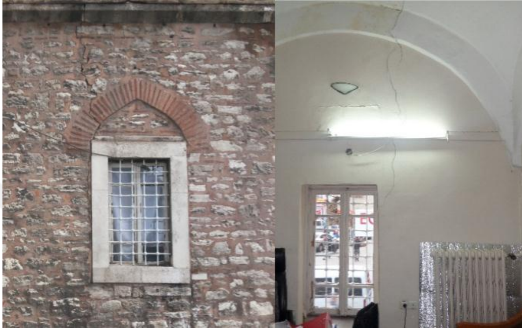
Figure 5.35: Damage of wall (G10F11) 1. Exterior Face of Wall 2. Interior Face of Wall
