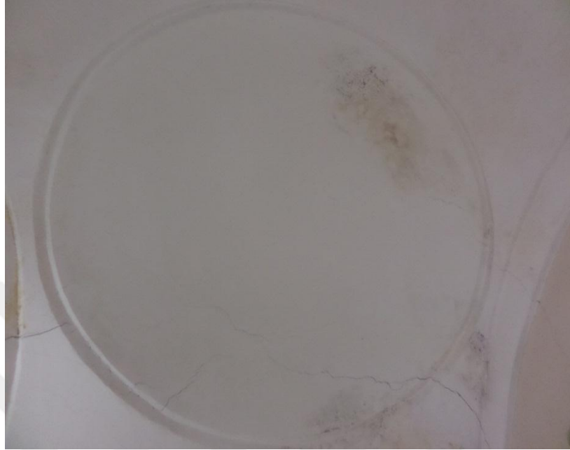
Figure 5.9: Damage of Dome (G10G11F10F11)
