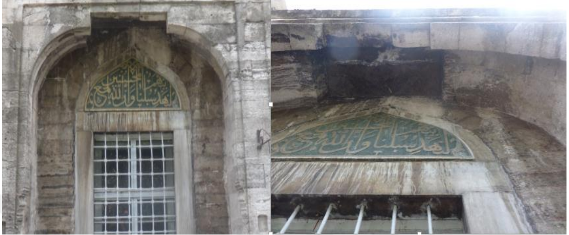
Figure 5.23: Damage of Bursa Arch (G4G6H4H6)
