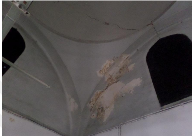
Figure 5.19: Damage of Pendentives on the main Classroom (I5I7F5F7)
