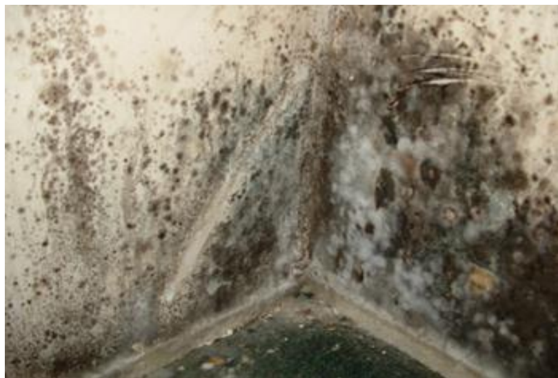
Figure 3.2: Spots and Patches on a Wall Due to Fungus
