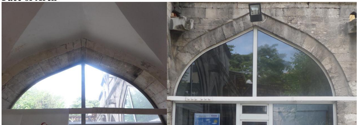
Figure 5.14: Damage of Arch (E8E10F8F10) 1. Interior Face of Arch 2. Exterior Face of Arch
