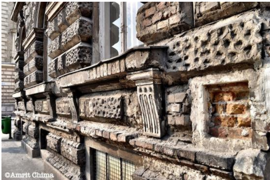
Figure 3.6: Building Decay Caused by Pebbles in Hungary
