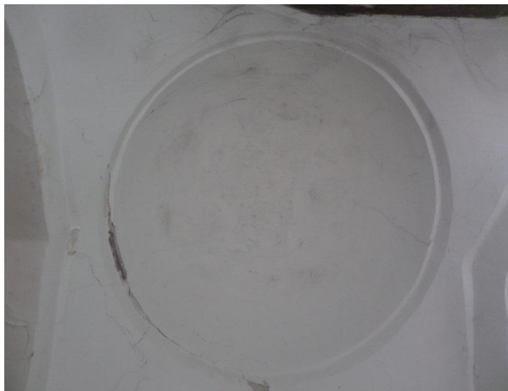
Figure 5.2: Damage of dome (A6A7B6B7)
