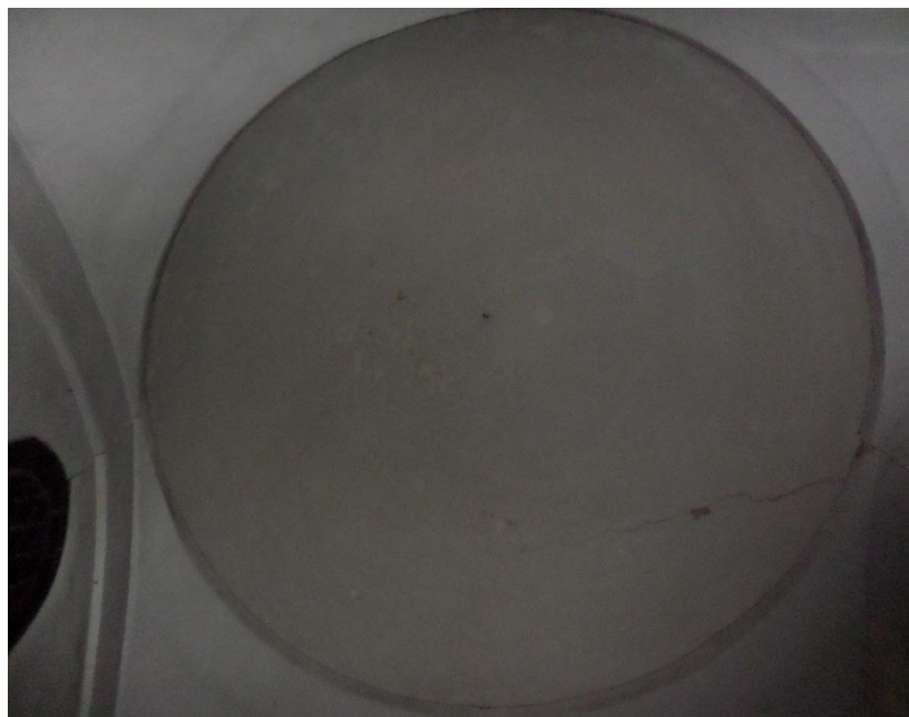
Figure 5.6: Damage of Classroom Dome (I5I7F5F7)
