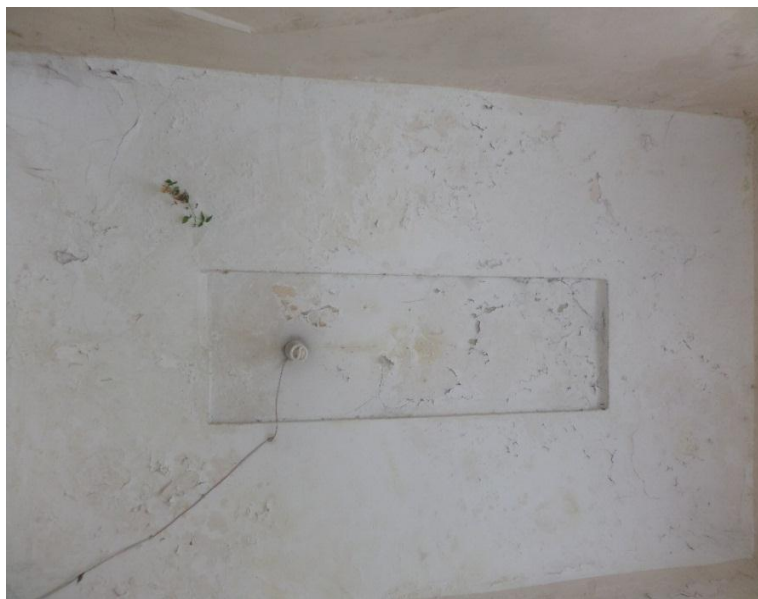
Figure 5.12: Damage of Ceil of side Entrance
