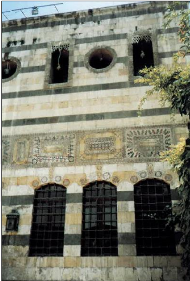
Figure 4.49: The Lower Windows of Qaa inside Al-Azem Palace Protected with Iron Blusters
