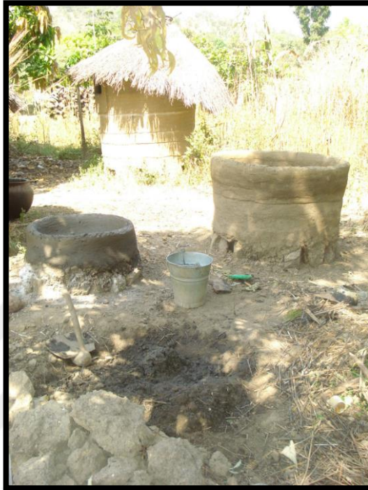
Figure 0.5: The erection of the walls of a grainary using the build in-place method
