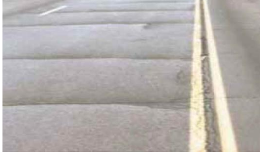
Şekil 3.31. Enine Çatlaklar (California Department of Transportation, 2001)
